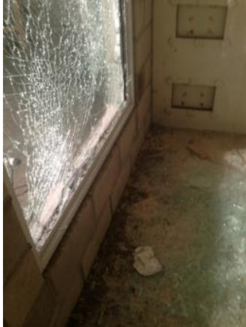
Figure 3.7: Failure of unprotected outer glass
