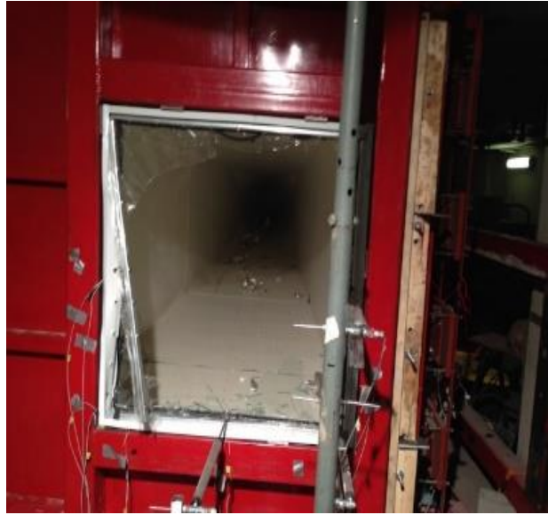
Figure 3.11: Failure of a window frame
