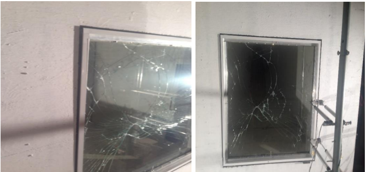
Figure A.14: Photographs of C7 after testing
