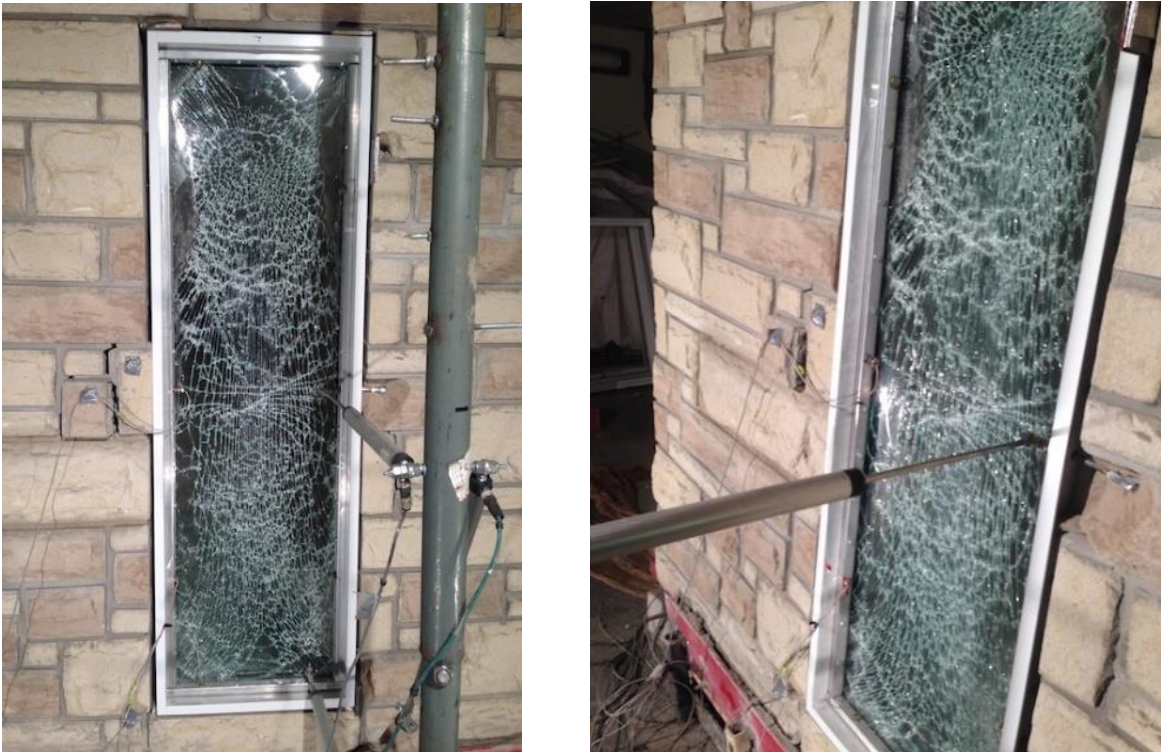
Figure B.36: Photographs of window after Test ST6
