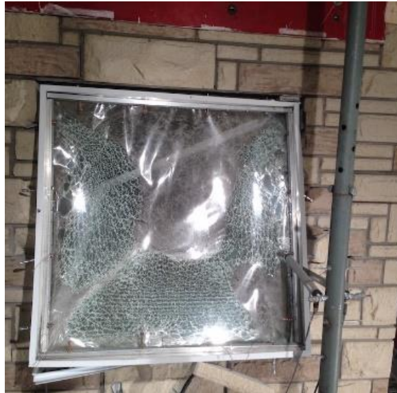
Figure 3.13: Square window on stone masonry after the application of 69 kPa
