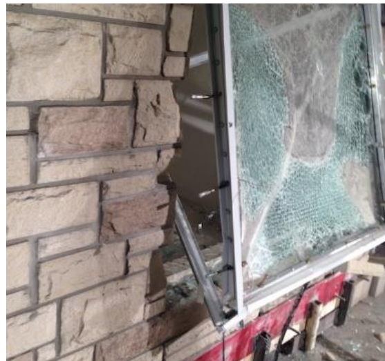
(b) Stone wall after test ST2
