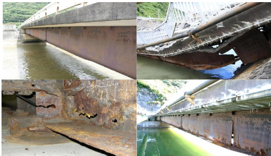
Figure 1- 1: Plate girder bridge in Japan experiencing structural failure (Kim et al., 2012)
