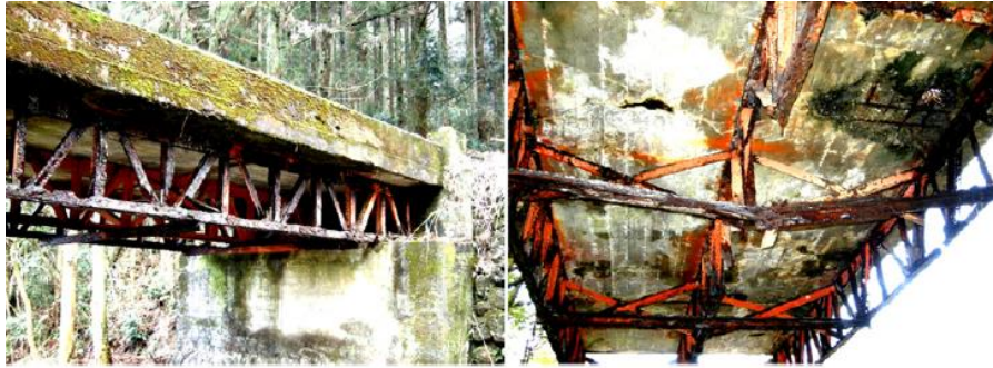
Figure 1- 2: Steel truss bridge in Japan experiencing structural failure (Ahn et al., 2014)
