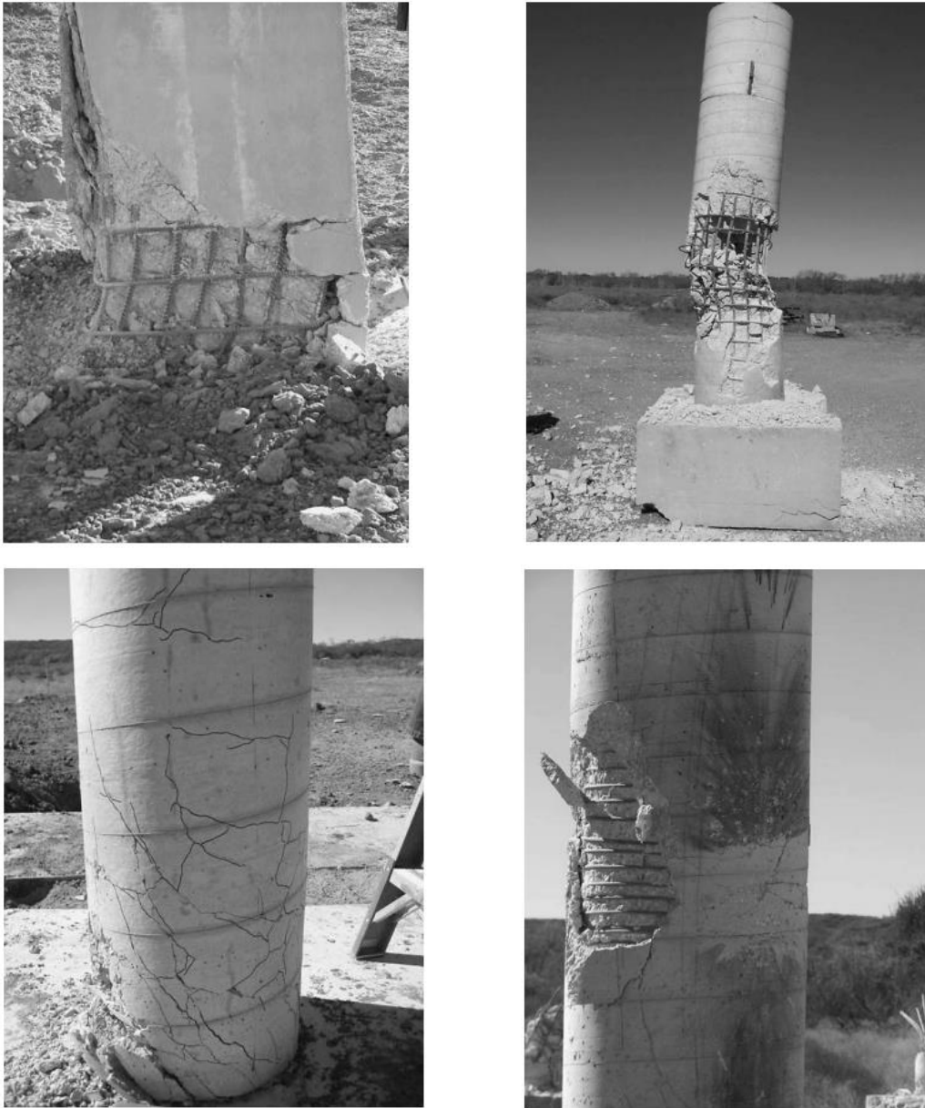
Figure 2-17: Observed Modes of Failure during NCHRP Project (NCHRP Report 645 2010)
