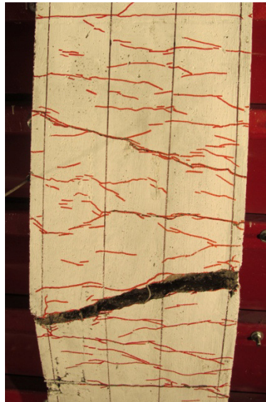
g) Mid-span cracking at Blast 5
