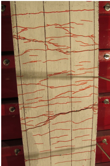
f) Mid-span cracking at Blast 3
