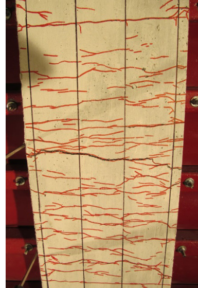
c) CRC-2%A-#3SS-100 Tensile cracking after Blast 5
