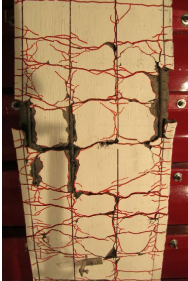
a) SCC-0%-#3NS-100 Damage at Blast 4
