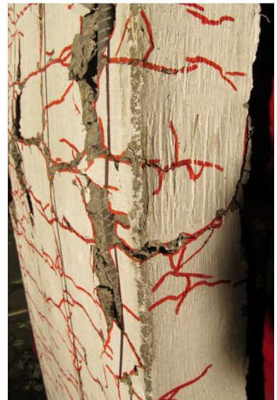
h) Mid-span cracking at Blast 5
