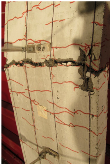
e) Mid-span cracking at Blast 3
