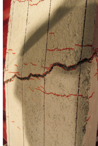
b) CRC-2%B-#3NS-80 Tensile cracking after Blast 3
