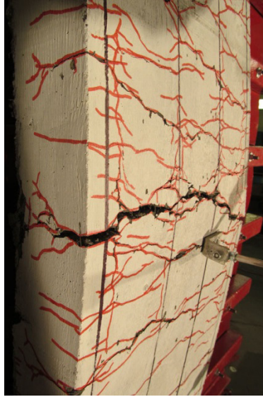
b) SCC-0.6%BP-#3NS-100 Damage after Blast 4
