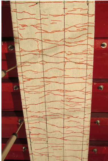
a) CRC-2%A-#3HS-100 Tensile cracking after Blast 5
