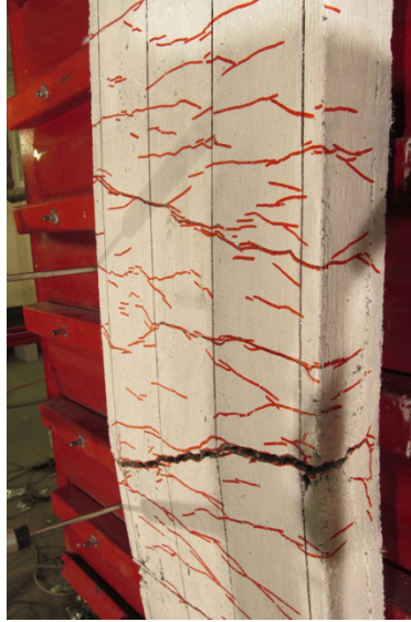
b) CRC-2%A-#3NS-100 Tensile cracking after Blast 4
