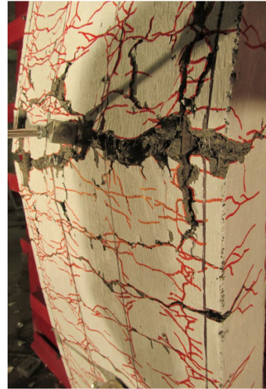
h) Exposed rebar at Blast 5
