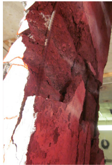
h) Exposed compression steel at Blast 5
