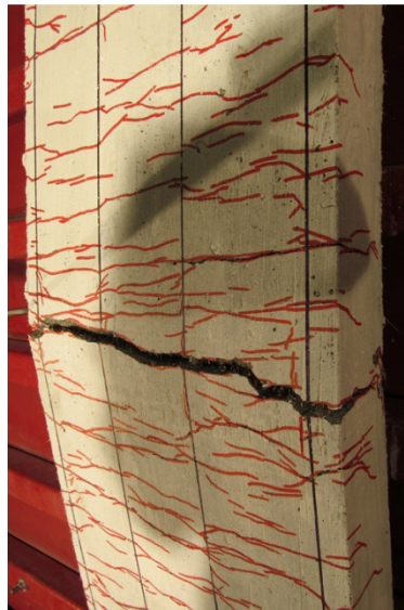
h) Mid-span cracking at Blast 6
