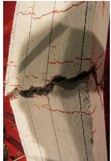
g) Mid-span cracking at Blast 4
