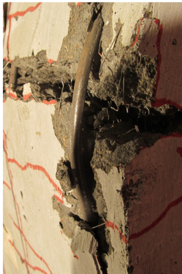
f) Bar slippage at Blast 4
