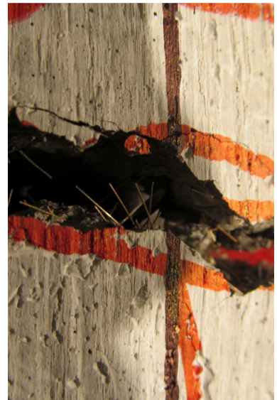
i) Bar rupture at Blast 6
