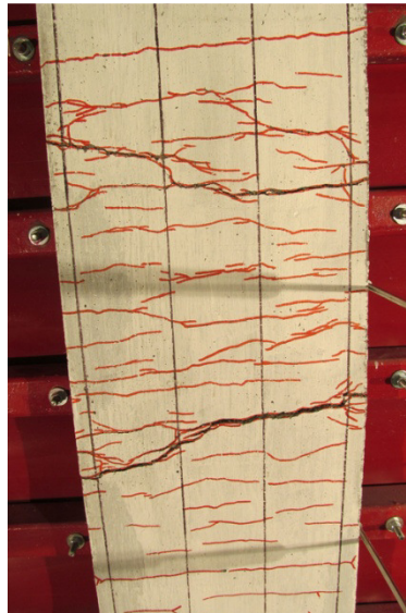
g) Mid-span cracking at Blast 4
