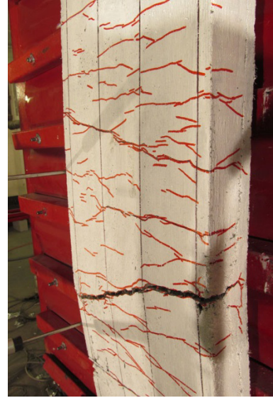
c) CRC-2%A-#3NS-100 Tensile cracking at Blast 4
