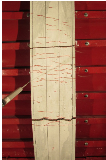
f) Mid-span cracking at Blast 4
