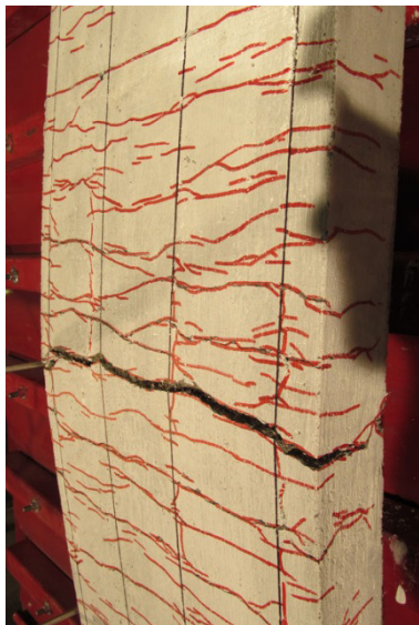
d) CRC-2%A-#3HS-100 Bar rupture failure after Blast 6
