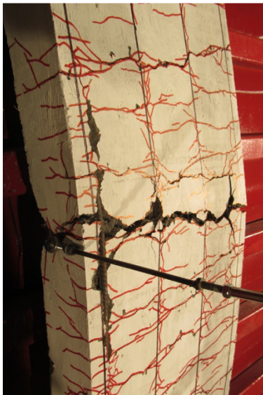
f) Mid-span cracking at Blast 4
