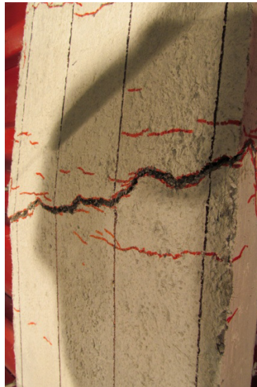
f) Mid-span cracking at Blast 3
