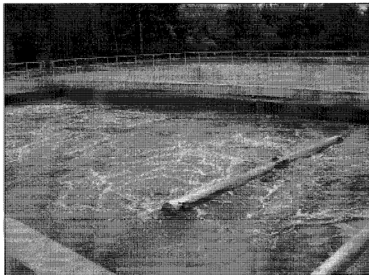
Figure 3.3: Contact basin at the Rockland, Ontario SBR facility
