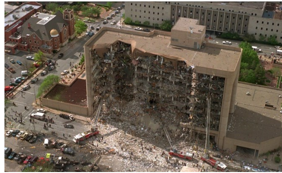
Figure 1.2: Former Alfred P. Murrah federal building in Oklahoma City, after the 1995 bombing (Murphy 2020)
