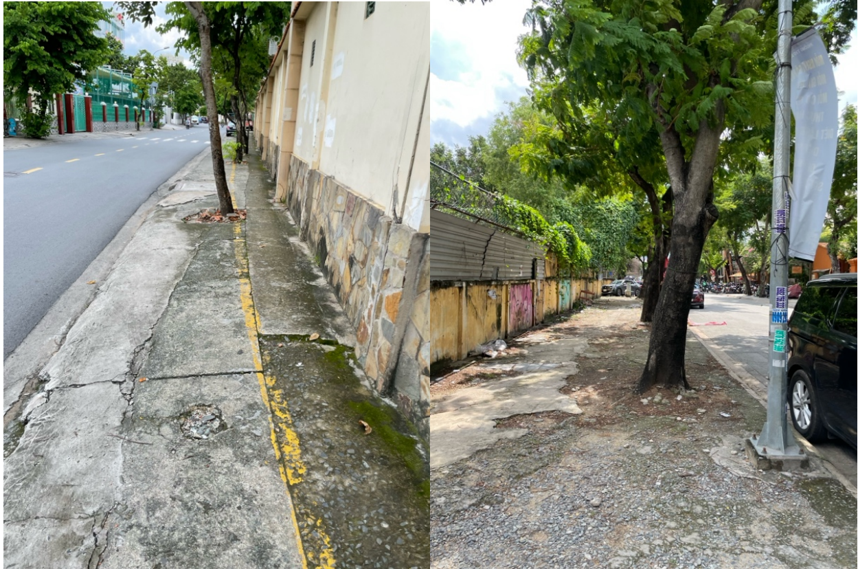
Figure 22: Broken sidewalks in residential districts in HCMC, 2022 (source: taken by author during 2022 fieldwork)
