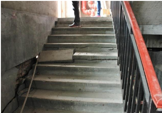
(c) Damage on the Staircase at First Floor
