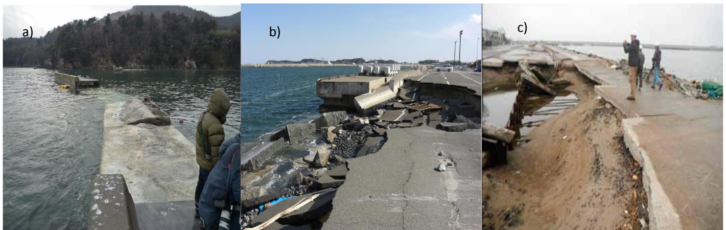
Figure 1.2: Destruction of port infrastructures by the 2011 Tohoku Tsunami a) Failure of breakwater at Takenoura, Onagawa Town.(Mikami et al., 2012) b) Damage of wharf at Soma Port.(Mikami et al., 2012) c) Scour around the quay support sheet pile. (EERI, 2011)
