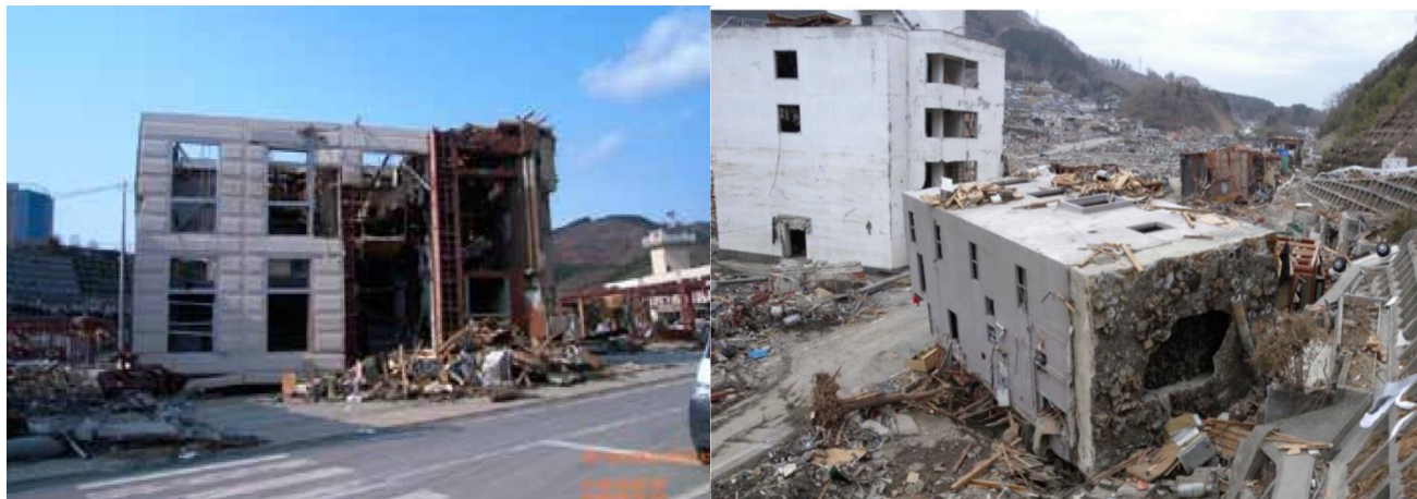
Figure 1.4: Destruction of inland building due to tsunami-induced hydrodynamic forces and overturning moments (a) Steel-frame building [Courtesy of Chock] (b) Reinforced concrete building [Courtesy of Koshimura].2011 Tohoku Tsunami, Onagawa city, Miyagi prefecture, Japan
