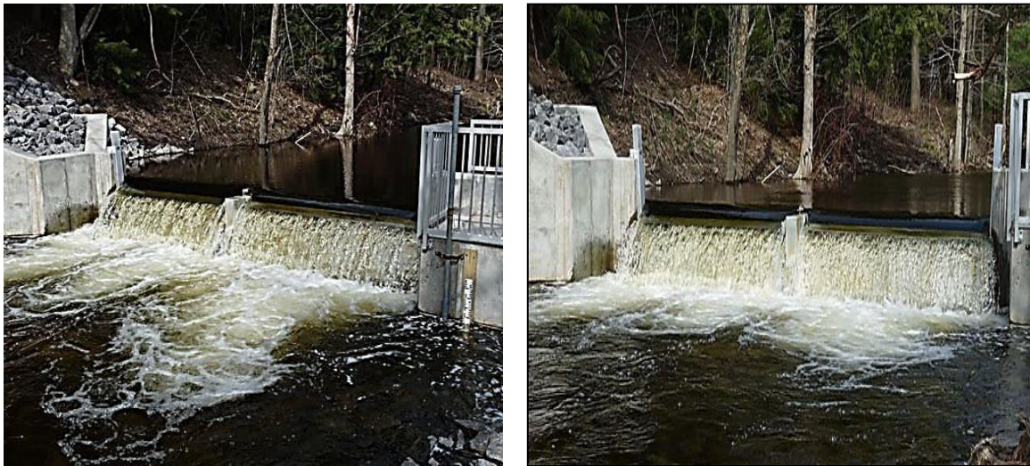
Figure 1-1: Sea lamprey barrier built in Pulaski, NY in 2013. Courtesy of the Department of Fisheries and Oceans (Government of Canada).
