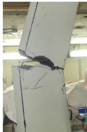
g) Mid-span cracking right side (Blast 4)
