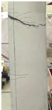
f) Mid-span cracking right side (Blast 4)
