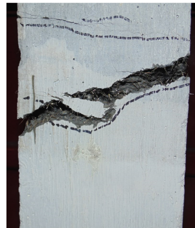
g) Mid-span cracking close-up on tension side (Blast 4)
