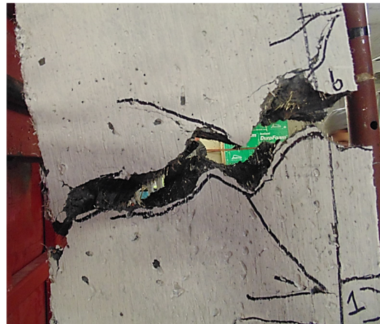
g) Mid-span cracking close up (Blast 4)
