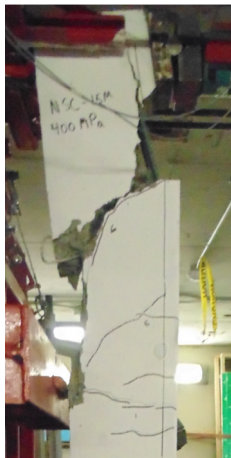
d) Shear Failure (left side) (Blast 3)
