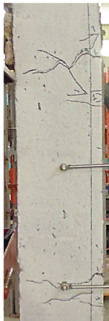
e) Mid-span cracking (Blast 3)
