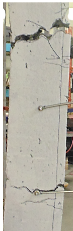
f) Mid-span cracking (Blast 4)
