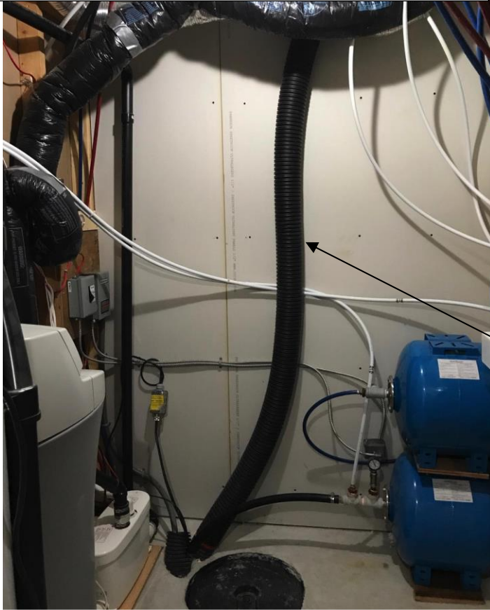
e. SDSS after installation (inside)
