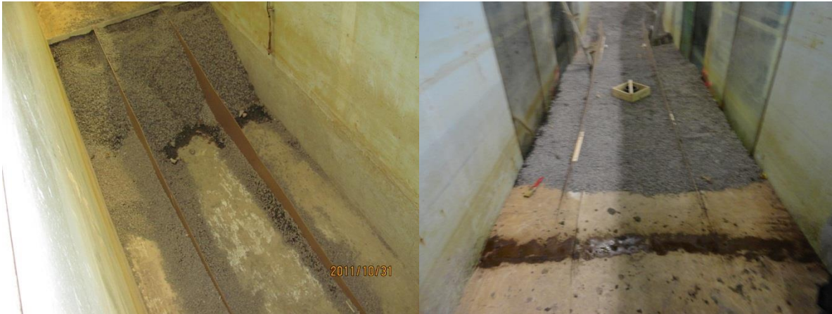
Figure 3.12: Left: Formwork for bathymetry transitioning from deep to shallow water; Right: Gentle slope bathymetry formwork in shallow water zone with formwork for level pad at location of the structure
