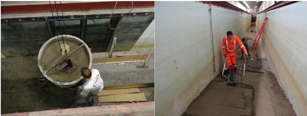
Figure 3.13: Pouring concrete through use of a crane and bucket (left); Troweling concrete on foreshore (right)
