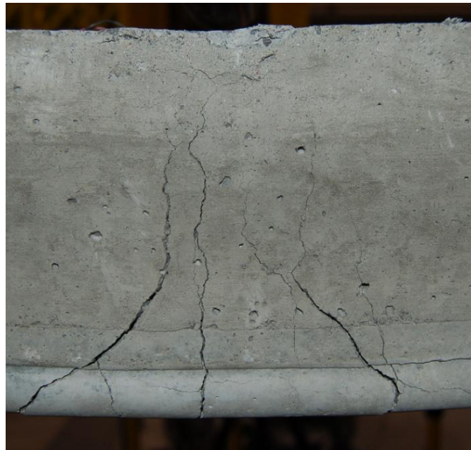
Figure 4-7: Midspan zone damage in Imp-2 (lower edge rounded and indented for this specimen due to prototype formwork modifications)
