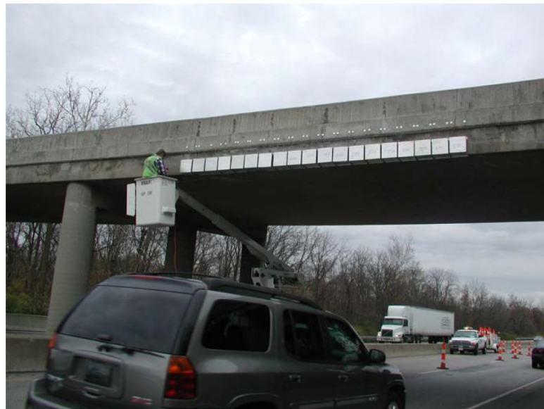
Figure 2-28: Field installation of I-Lam panels on concrete bridge (DEL-23-12.99) in Delaware, U.S. (Qiao et al., 2008)
