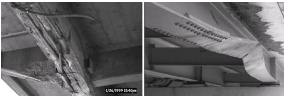
Figure 2-25: Damage to concrete and steel bridge girders resulting from overheight vehicular impacts (Sharma et al., 2008)
