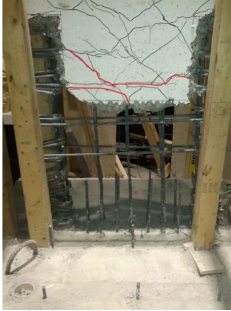
Figure 3.14: Inclined Crack in Wall RW1-SR
