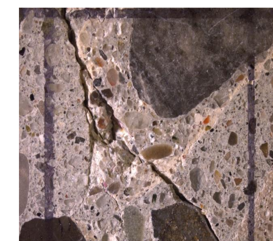
The crack splits into a fork within the residual mortar
