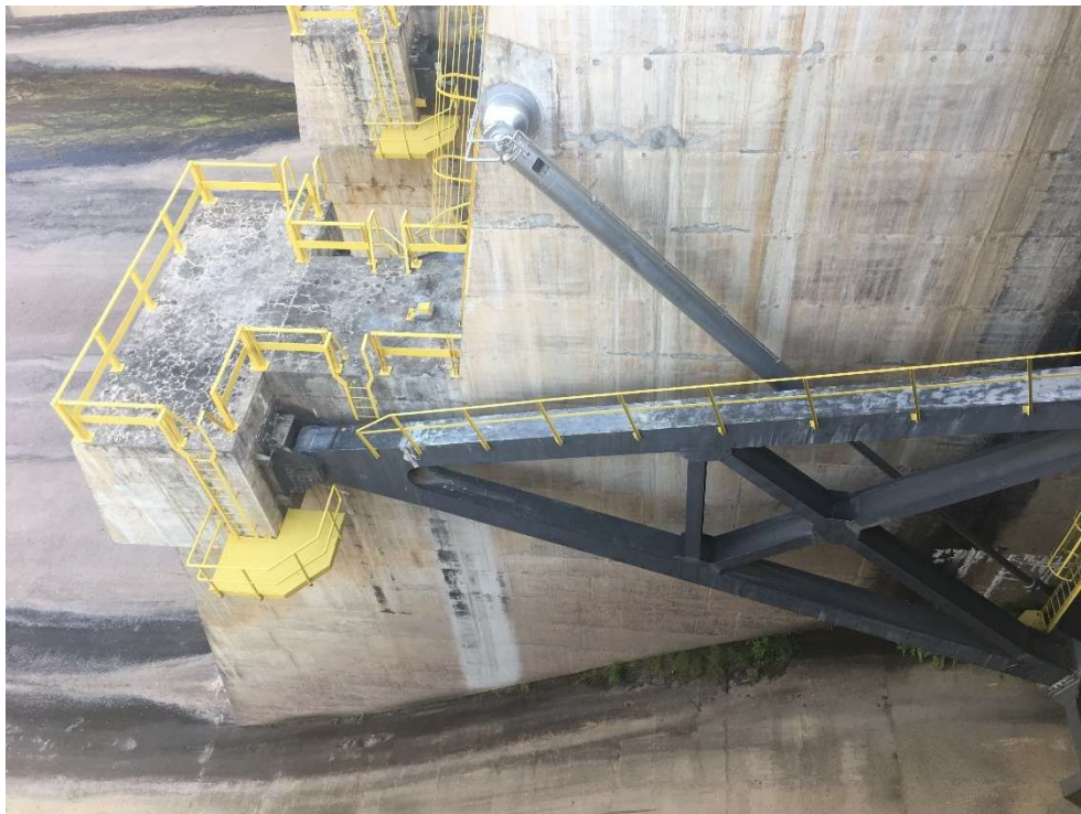
Figure 4-1. Paulo Afonso IV dam - Spillway: a. Overview, b. Close-up of the ASR damage.
