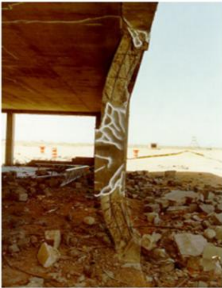
(a) Failed unreinforced column (DB 6)
