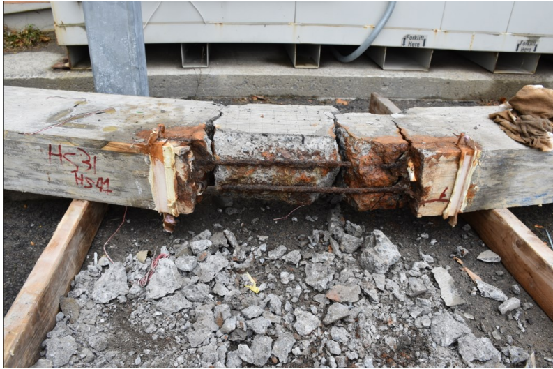
Figure A.85: Corrosion-induced damage in the cover of concrete – beam SS-4.1
