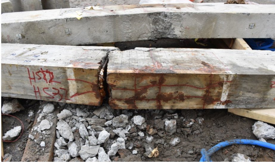
Figure A.67: Corrosion-induced damage in the cover of concrete – beam SS-3.2
