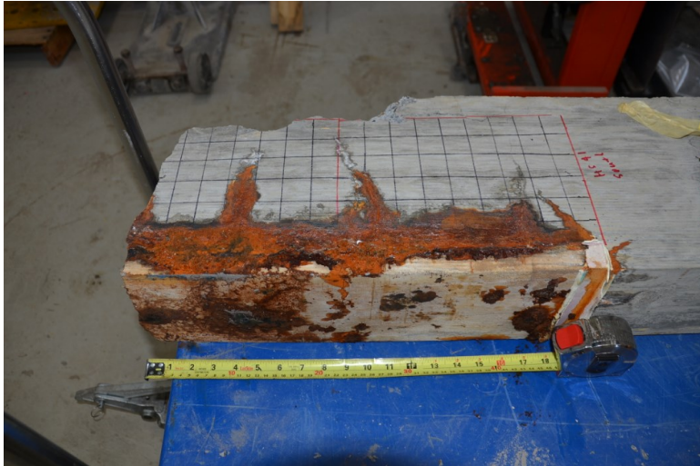
Figure A.33: Corrosion-induced damage in the cover of concrete – beam SS-2.2
