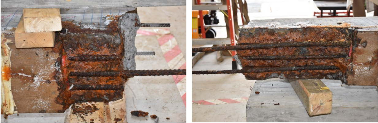
Figure B.43: Corrosion-induced damage in the cover of concrete – beam LS-2.2
