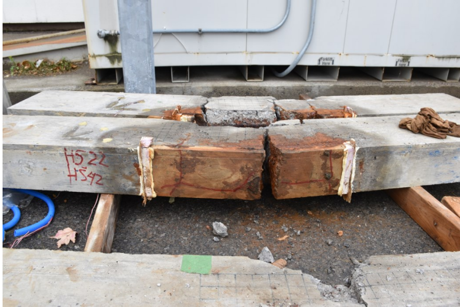
Figure A.103: Corrosion-induced damage in the cover of concrete – beam SS-4.2
