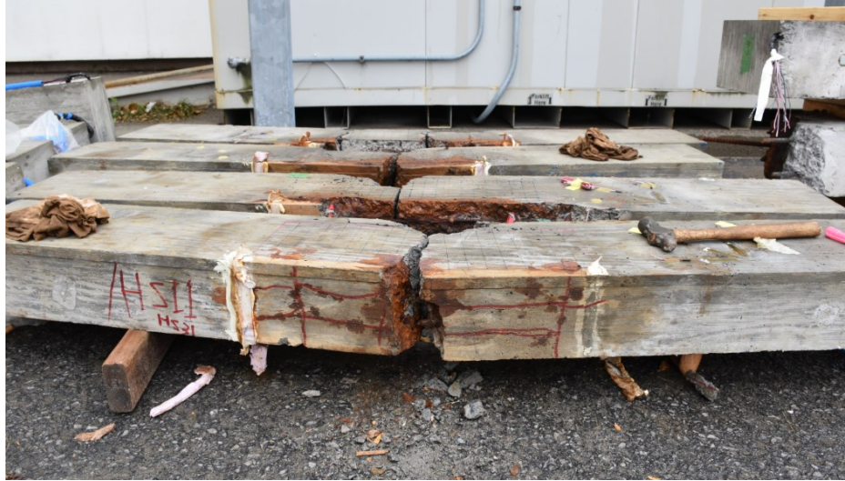
Figure A.49: Corrosion-induced damage in the cover of concrete – beam SS-3.1
