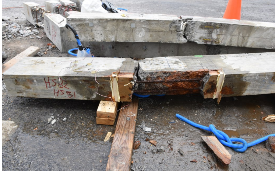
Figure A.121: Corrosion-induced damage in the cover of concrete – beam SS-5.1
