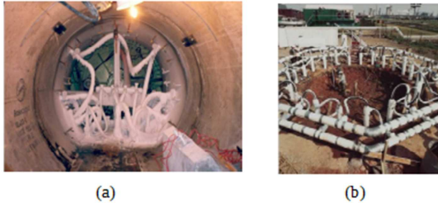
Figure 16: Ground freezing tubes used to excavate (a) tunnel (Frank Coluccio Construction, 1996) and (b) shaft (BDF, 2009)
