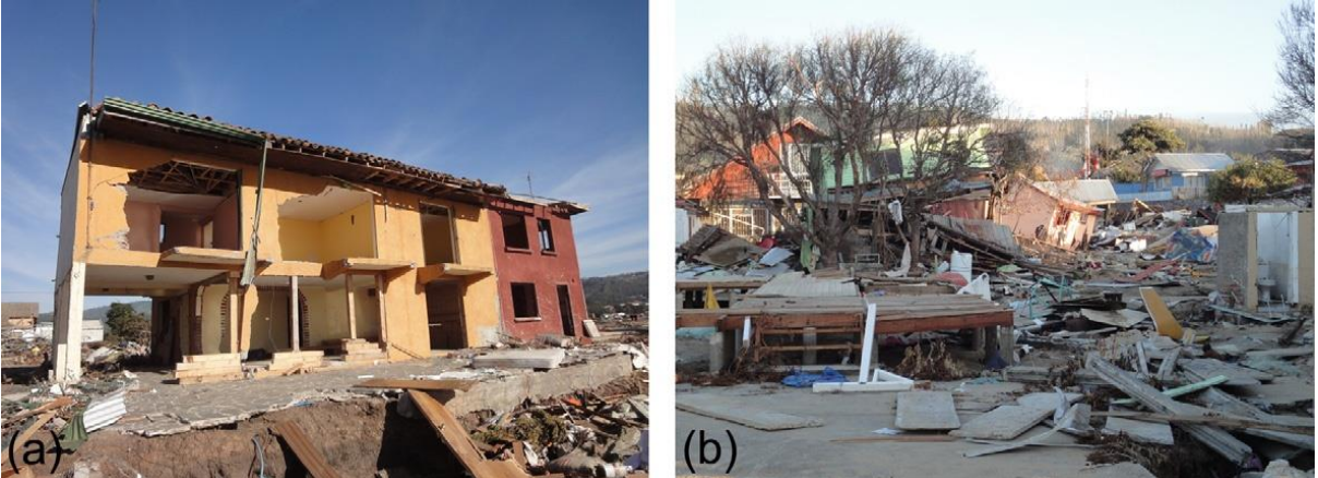
Figure 2-12 Tsunami damage due to the February 2010 Chile Tsunami. (Nistor and Palermo 2015)
