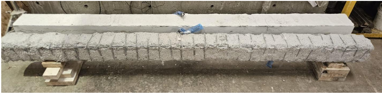
Figure 3.29 – Photos showing the process of roughening the surface of the column on all four sides prior to pouring ECC jacket.
