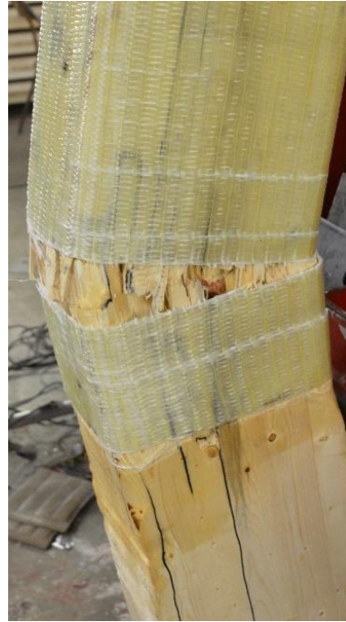
(b) Close-up of damage for D3.1
