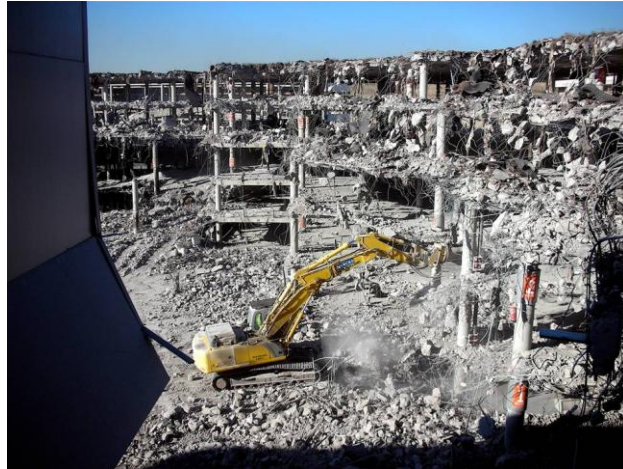
Figure 2.1 Effects of the 500kg explosive on the RC parking structure of Terminal 4
