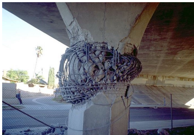
Figure 1-1 Typical concrete column failure due to poor confinement
