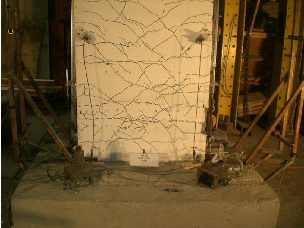
Figure F.42 W1-SR Wall After (1.5%) Drift
