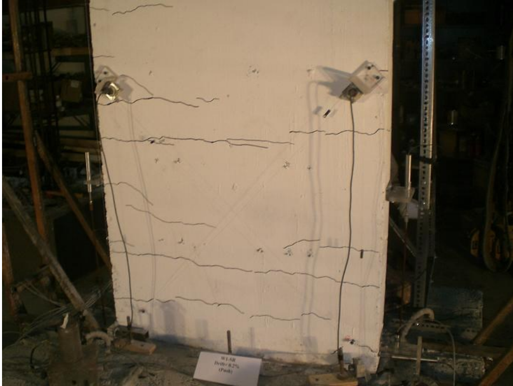
Figure F.36 W1-SR Wall After (0.2%) Drift
