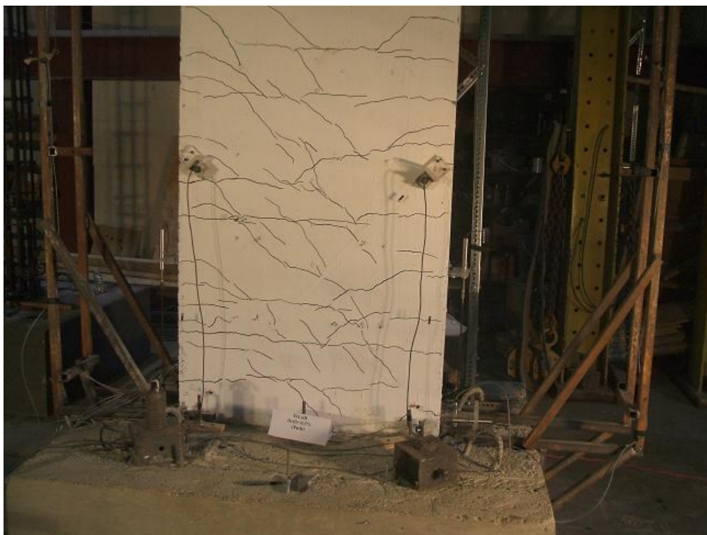
Figure F.38 W1-SR Wall After (0.5%) Drift
