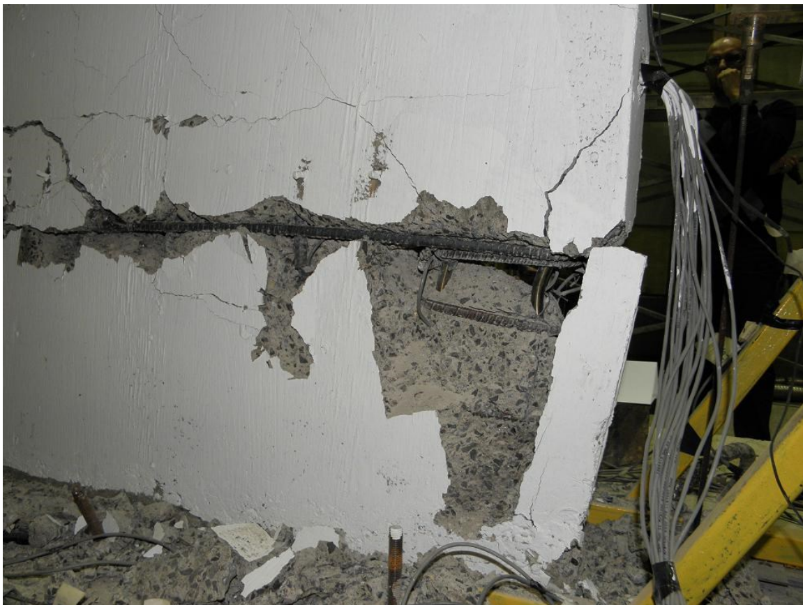
Figure 4.23 SMA Shear Wall Condition at Displacement Level of 108 mm (Failure)
