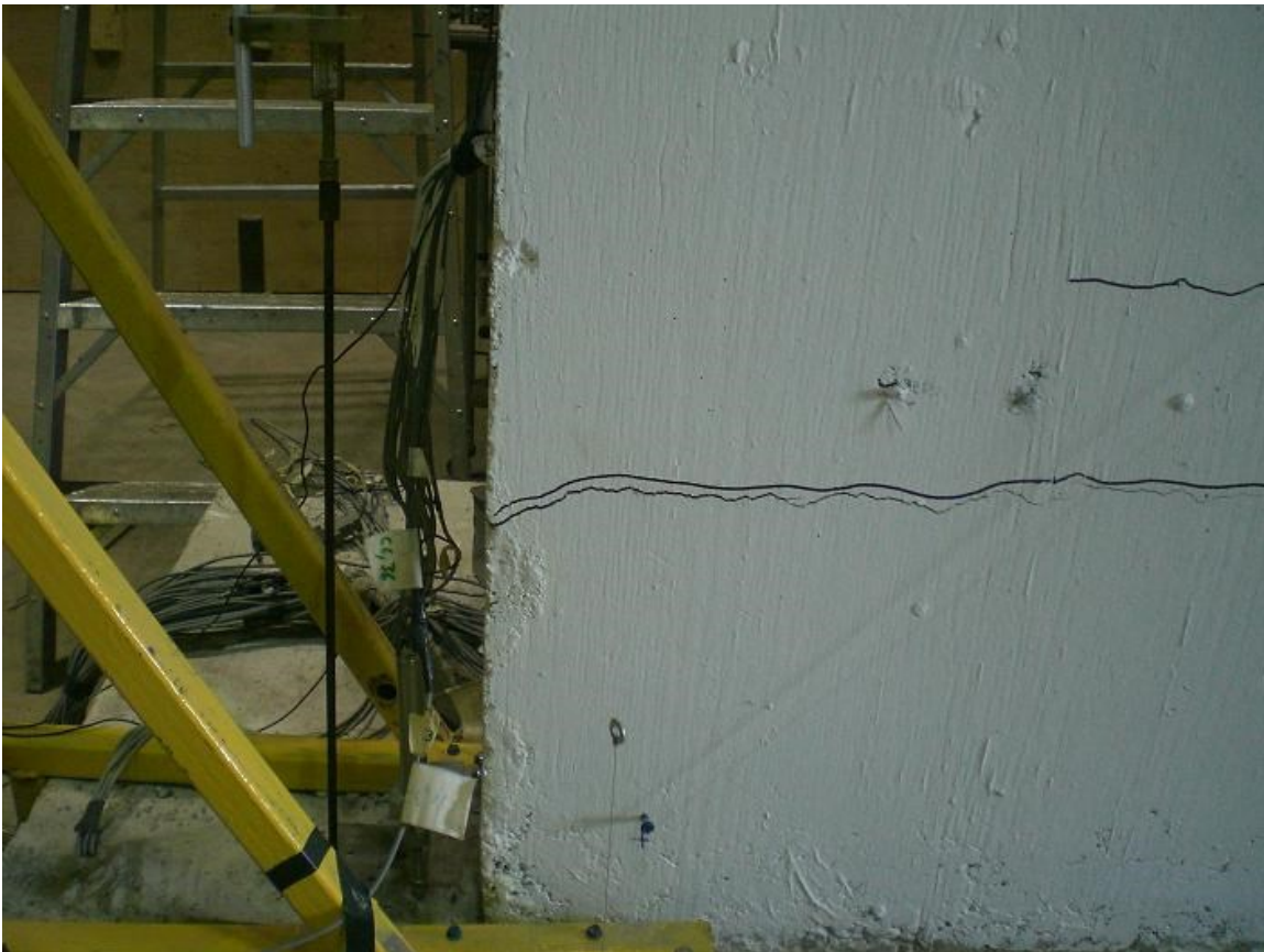
Figure 4.15 Flexural Crack in SMA Shear Wall
