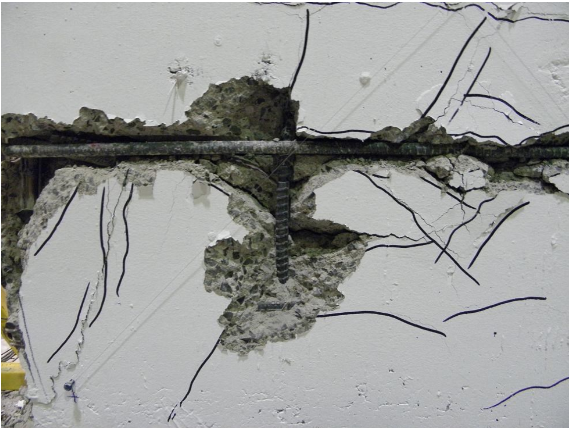
Figure 4.22 SMA Shear Wall Condition at a Displacement Level of 72 mm
