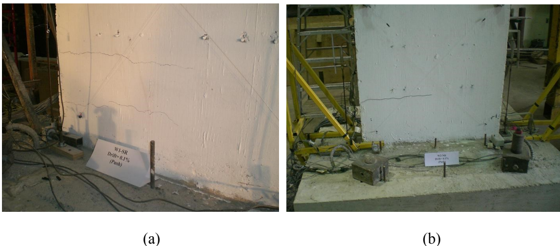
Figure 4.14 First Flexural Cracking in Shear Wall Specimens: (a) W1-SR; and (b) W2-NR
