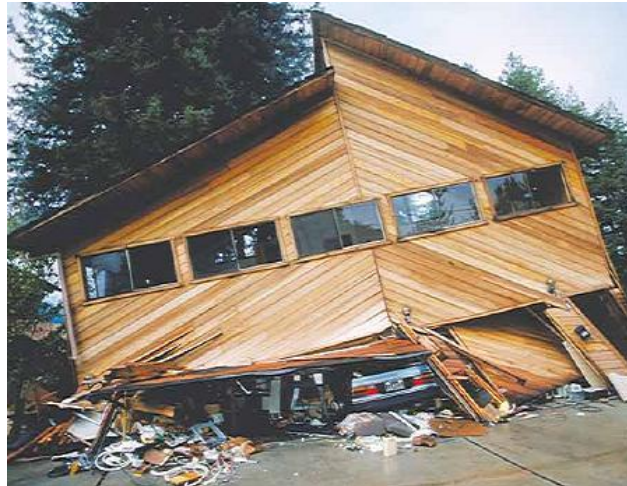
Figure 1-1: A light wood frame building in Santa Cruz Mountains, California, collapsed in the 1989 magnitude 6.9 Loma Prieta Earthquake (Photo from USGS)
