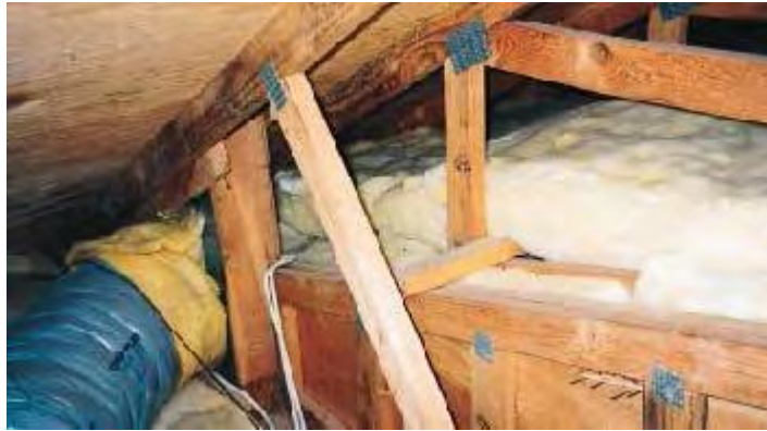
Figure 2-9: The Sheathing Panel on the Interior Shearwall not extended to the Roof Diaphragm (Fowler, 1998)
