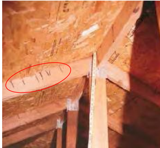
Figure 2-8: Nails Missing the Truss (Fowler, 1998)
