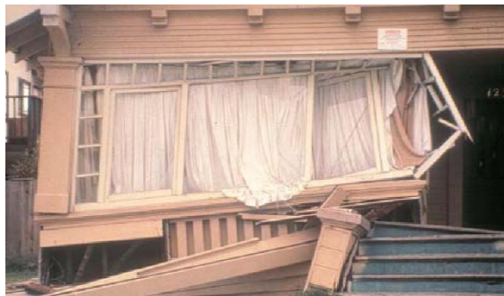
Figure 2-5: Failure of Cripple Wall in Loma Prieta Earthquake (Photo: C.Stover, U.S. Geological Survey)
