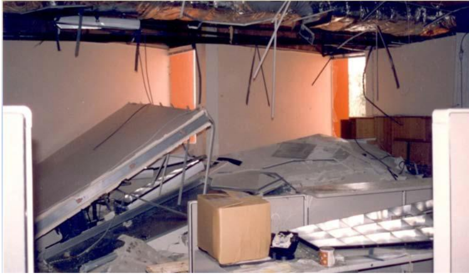
Figure 3-6: Failure of office partitions, ceilings, and light fixtures in the 1994 Northridge Earthquake (FEMA 74, 1994)
