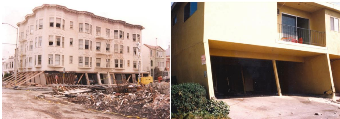
Figure 2-7: Failure in a Typical Wood Frame Construction Caused by Soft Story, in Loma Prieta Earthquake (Left) and Northridge Earthquake (right) (ATC, 2012)
