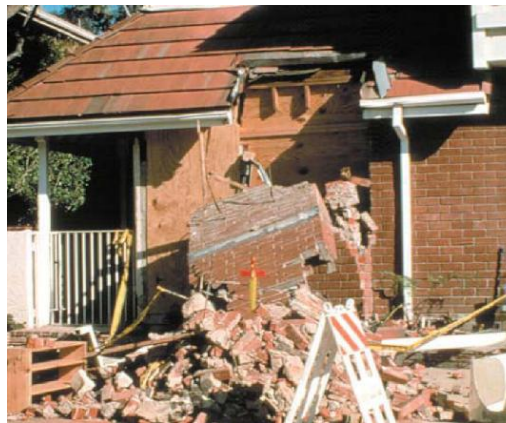
Figure 2-6: Chimney Damage in Northridge Earthquake
