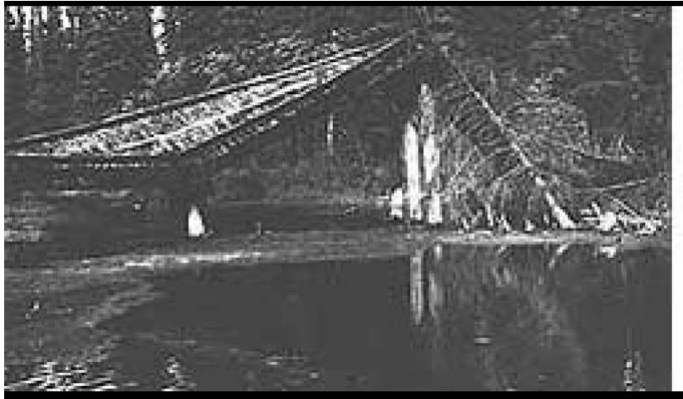
Figure 2.19 Piles at Clearwater Lake bridge in Alaska being forced out of ground due to frost heave (Pewe and Paige 1963)
