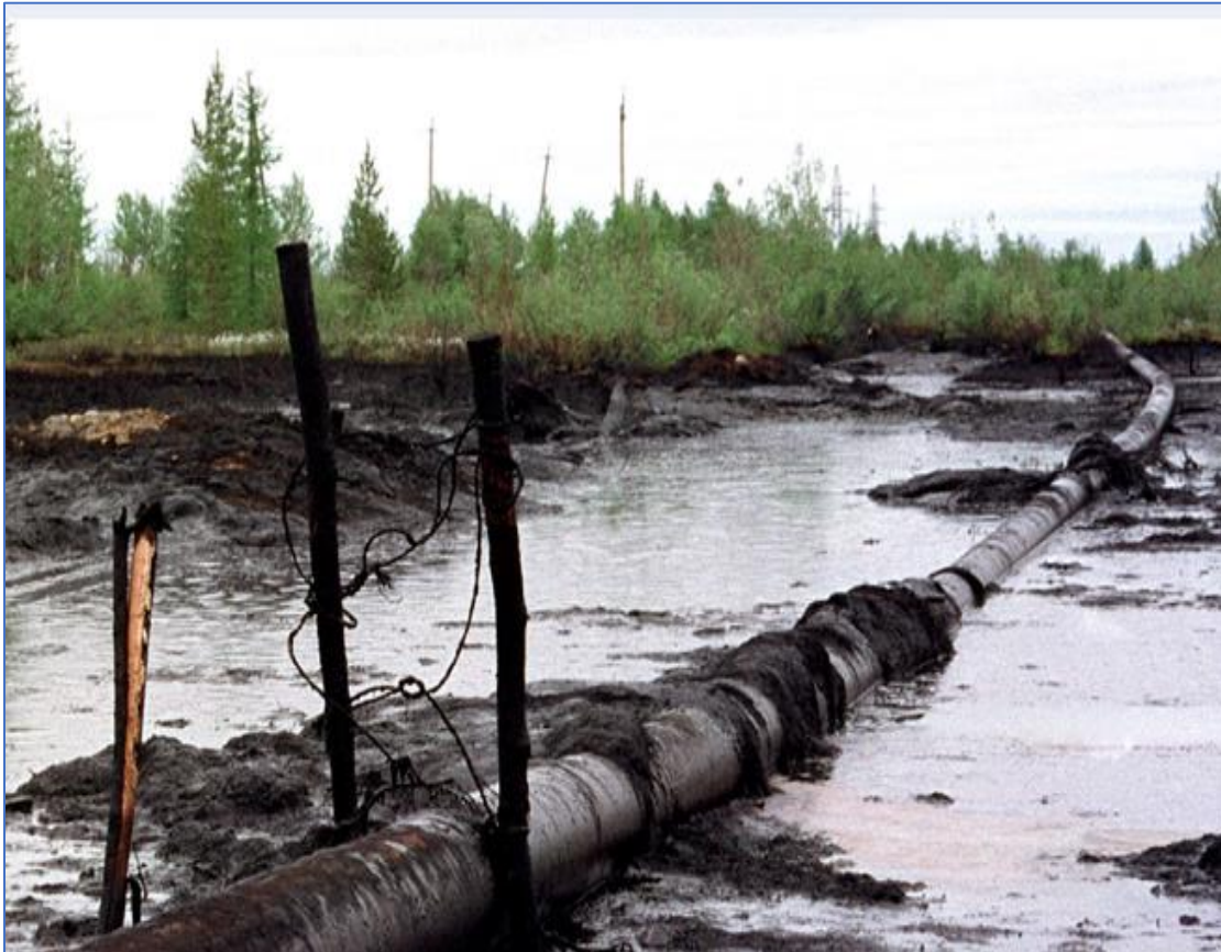
Figure 2.7 Thawing of permafrost threatens Russia’s oil and gas pipelines (Independent 2009)
