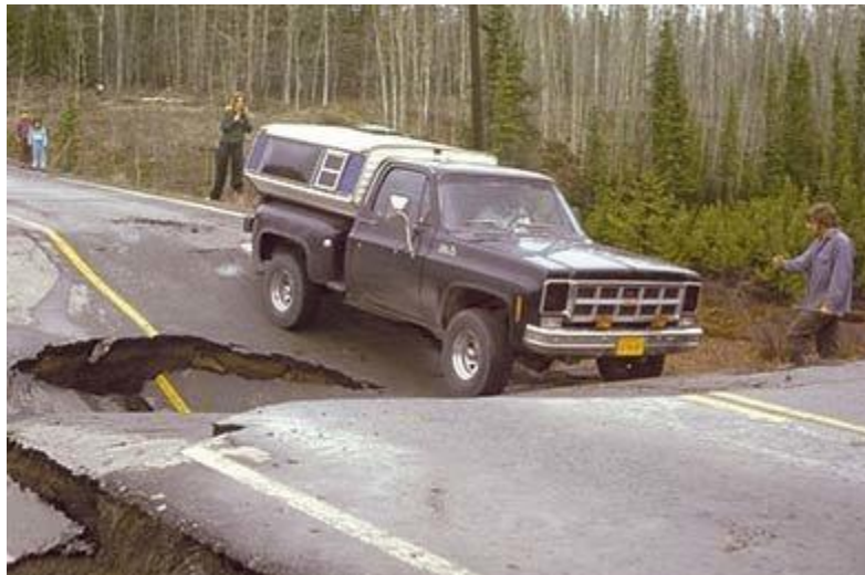
Figure 2.2 Permafrost damaged roads (Neill, 2011)
