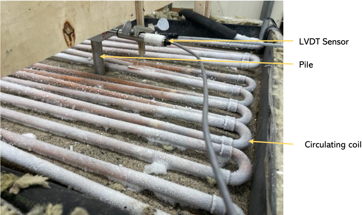
Figure B3 Soil freezing coils
