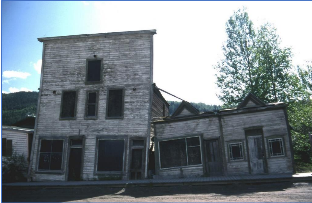
Figure 1.1: Building damage due to freezing and thawing of foundation soils (Shetler 2021)
