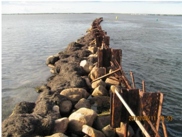
Figure 10.1 – 100 m long deteriorated structure at north end of the wharf.
