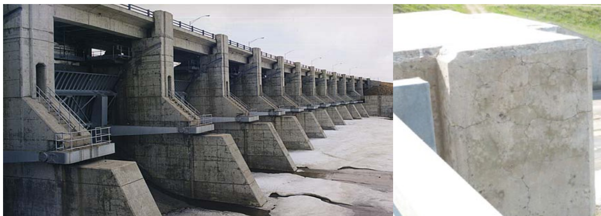
Figure 2.7: Gardiner dam spillway in Saskatchewan, Canada, showing map cracking (right) [59].
