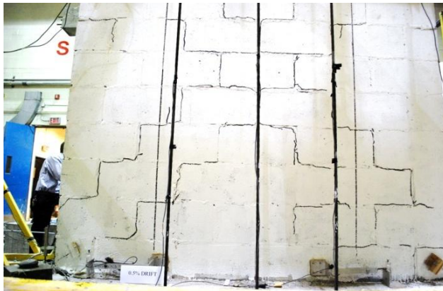
(c) Diagonal cracks at 0.5% drift
