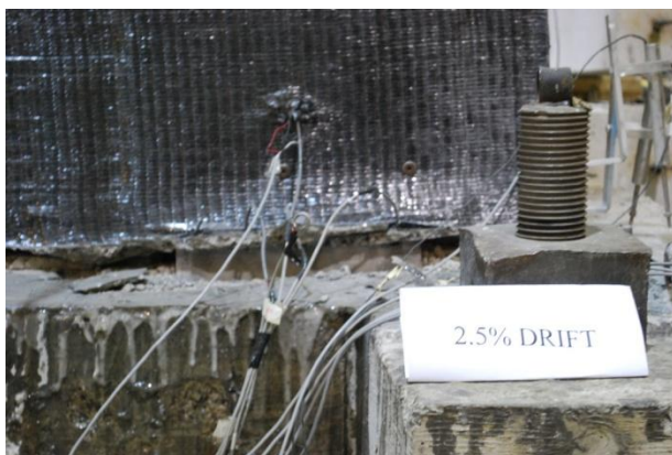
(c) Wall-foundation interface; 2.5% drift
