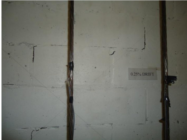
(a) Hairline diagonal cracks at 0.25% drift
