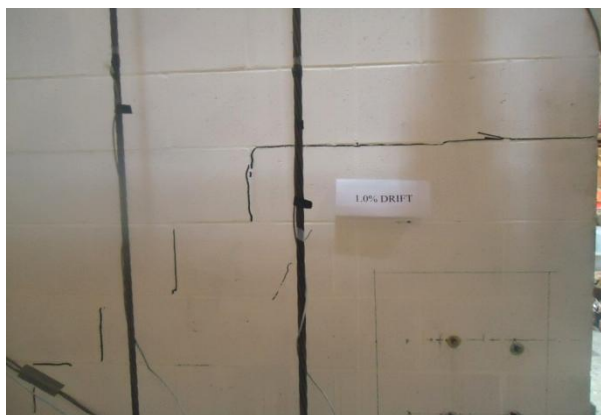
(a) Diagonal cracks at 1.0% drift
