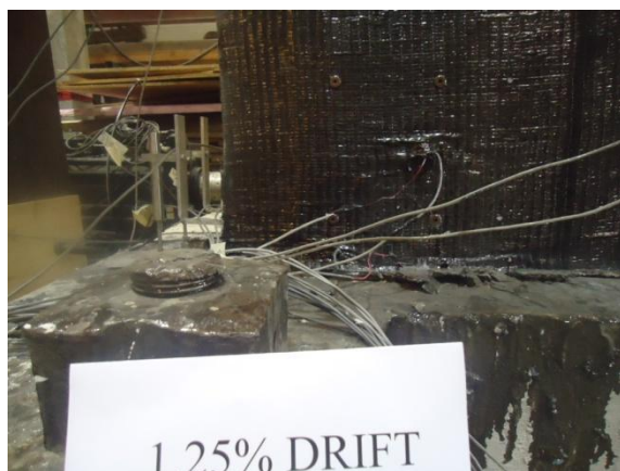
(e) Buckling of steel sheet anchor; 1.25% drift
