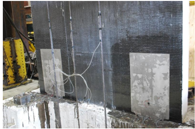
(b) Exposed anchors after adhesion
