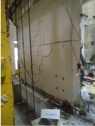
(a) Diagonal cracks at 1.5% drift
