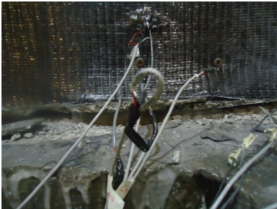
(e) Close-up view of anchor buckling; 1.5% drift
