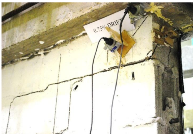
(e) Propagation of diagonal crack; 0.75% drift
