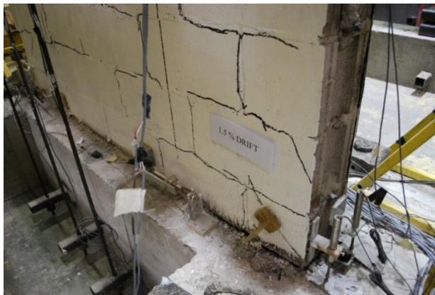
(e) Onset of crushing, west end; 1.5% drift
