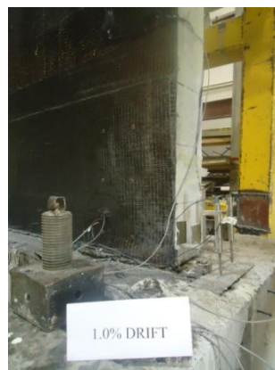
(b) Buckling of steel sheet anchor; 1.0% drift
