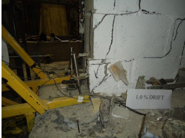
(a) Dislodged masonry block; 1.0% drift
