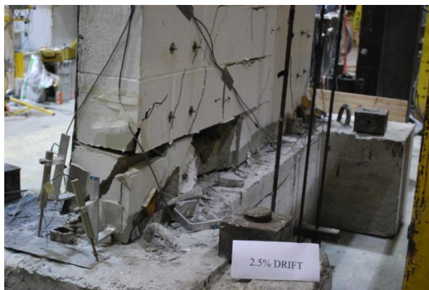
(a) Wall damage at east end; 2.5% drift
