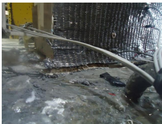
(f) Debonding of CFRP near the wall-footing interface; 1.25% drift
