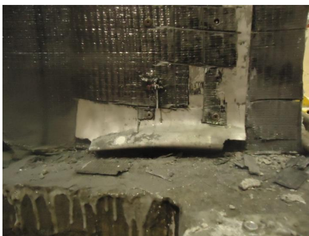
(e) Buckled steel sheet anchor after test (front view)
