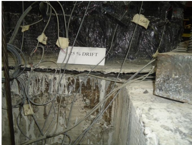
(c) Separation of FRP; 1.25% drift
