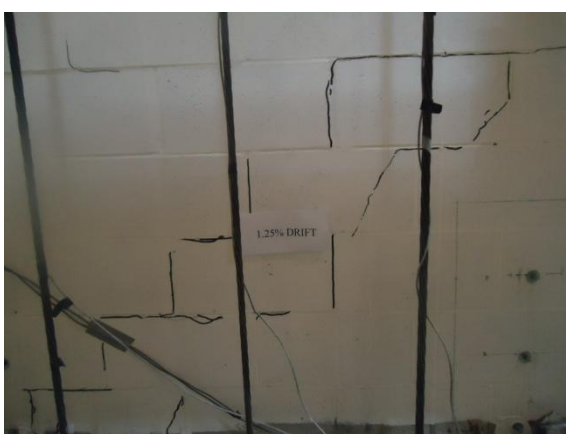
(c) Diagonal cracks at 1.25% drift
