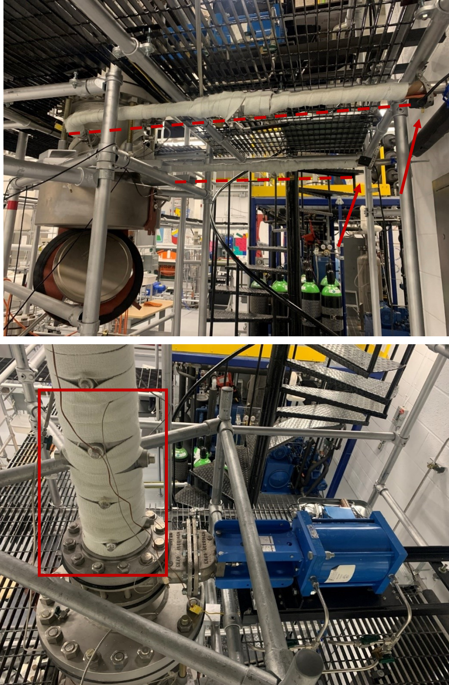
Fig. A - 3. Band heaters around the inlet pipes and the fluidization column
