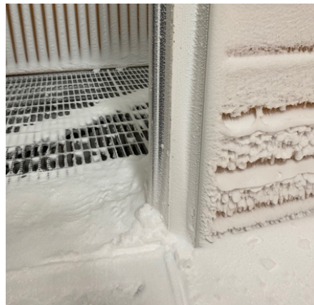
Figure 8 Snow building up in my door frame, causing the door to jam
