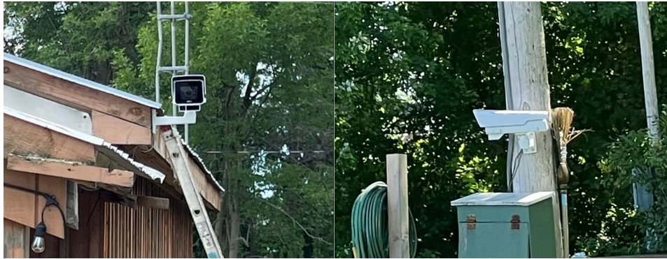
Fig. 5 Installed Axis cameras at Jacobs Island (left) and Mariatown Bay (right) for event-based wave and turbidity attribution.
