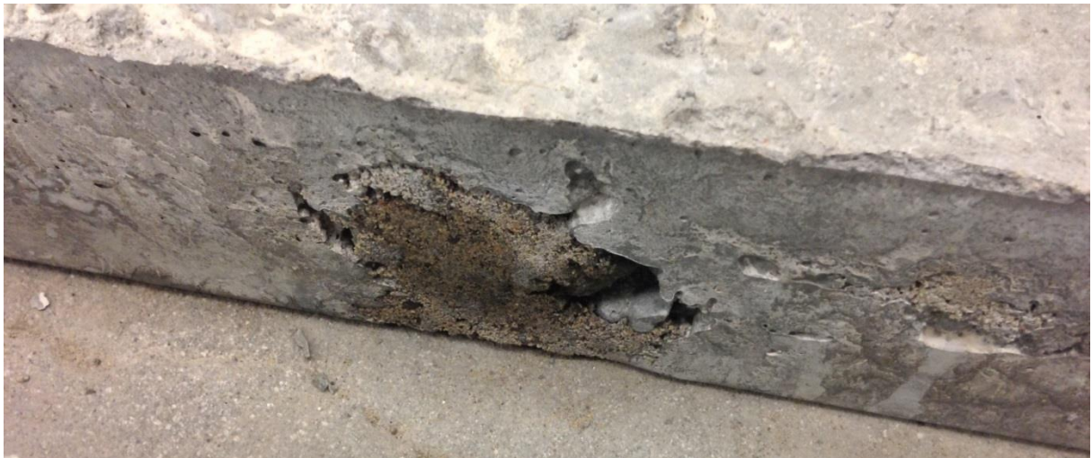
Figure 3.9: Poorly mixed concrete showing defects and large pores (batch 1a; w/c = 0.35 )
