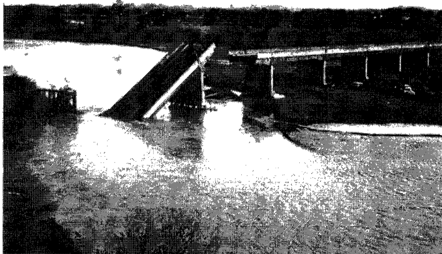
Figure 1-1 Bridge failure due to pier scouring - Bull Bridge on Rangitikei River, New Zealand, (1973). Breusers and Raudkivi (1991)
