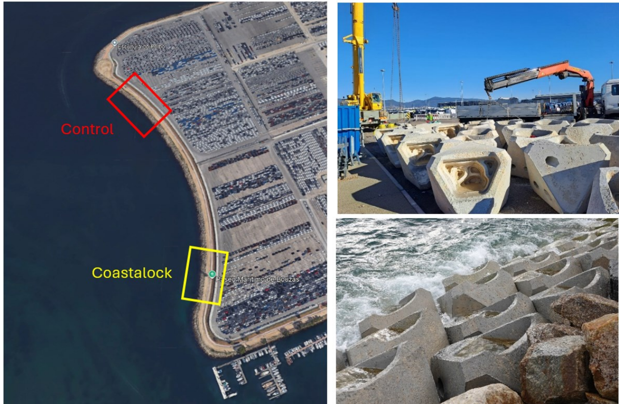
Figure 5-13. Left: Aerial view of the project's locations. Coastallock placement in Bouzas sloped protection; Right: Coastallock units after demoulding (upper) and after installation in Bouzas sloped protection (lower)
