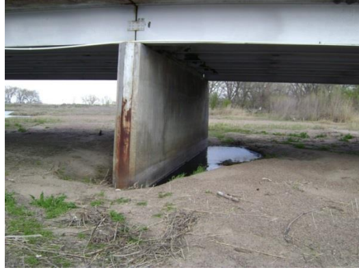
Figure 12: Scour Hole around a Bridge Pier on the Platte River, Nebraska (http://thestagnationpoint.blogspot.ca/)
