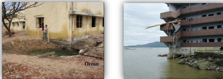
Figure 2: Tsunami-induced local scour at building foundations (Left: India (Yeh, 2004), Right: Japan (Nistor, 2012))
