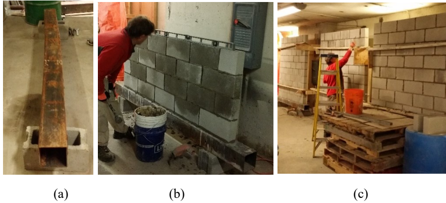
Figure 3-2. Construction of CMU wall; (a) Bed HSS, (b) Leveling of wall (c) Completion of the three walls and wood frame protection.
