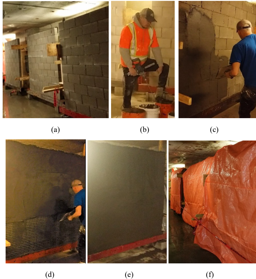
Figure 3-5. FRCM application; (a) Preparation of the surface, (b) Mixing of Mortar, (c) Base mortar layer (0.5 in thick), (d) Carbon grid layer, (e) Final mortar layer (0.5 in thick), (f) Walls curing with burlaps and plastic tarps.
