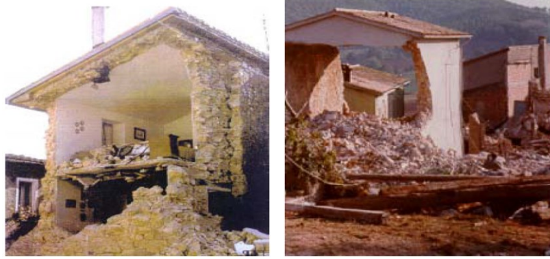
Figure 1-1. Out-of-plane failures of load-bearing URM walls during the Umbria Earthquake, Italy, 1997 (Babaeidarabad, 2013)
