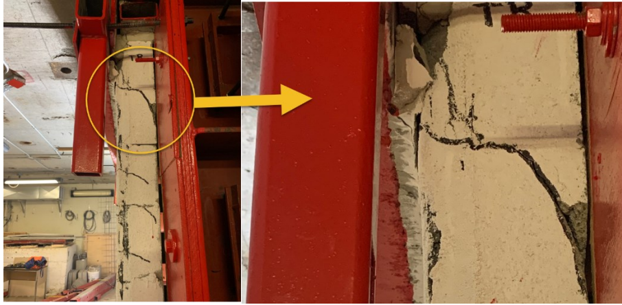
Figure 6-1. Out-of-plane shear demand on RCL-YC-3 after Blast ID #15
