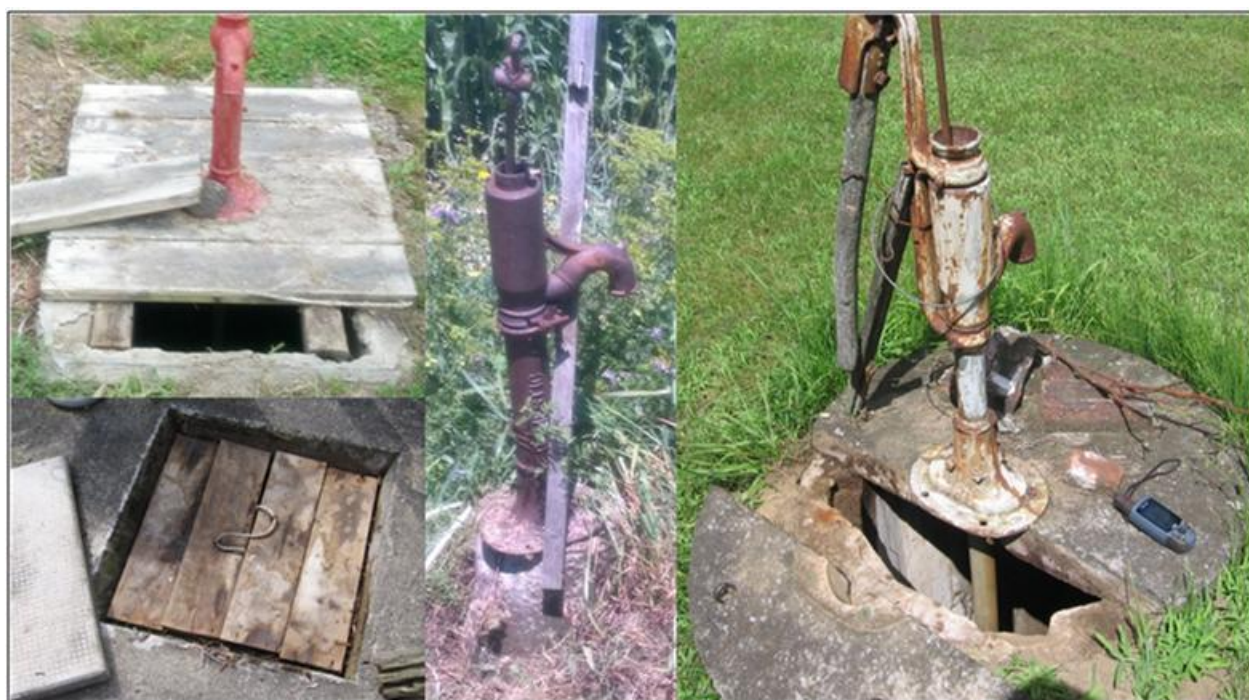
Figure 4-4. Wells encountered with improvised or otherwise old and damaged well covers.
