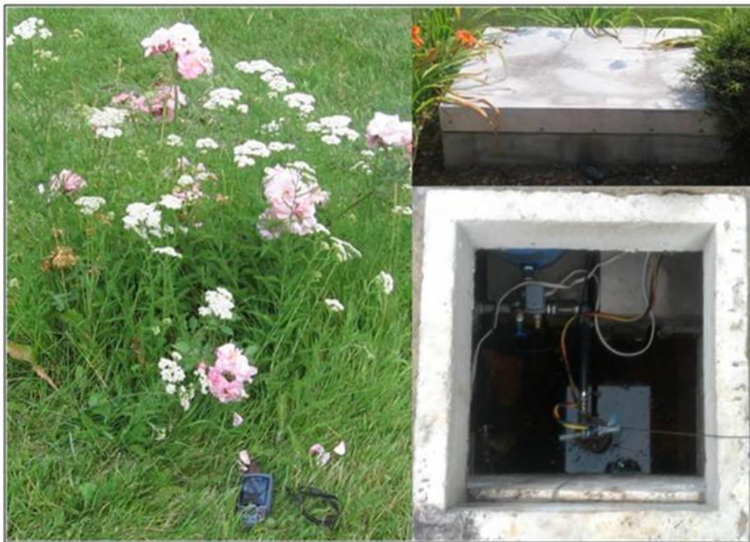
Figure 4-3. Wells encountered that were buried (left) or located in a well pit (right).
