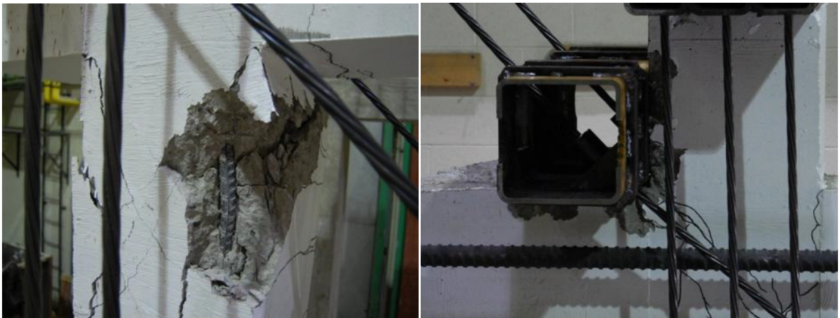
Fig. 4. 17 (a) Buckled longitudinal bar at the top of column, (b) localized crushing of concrete under bearing stresses
