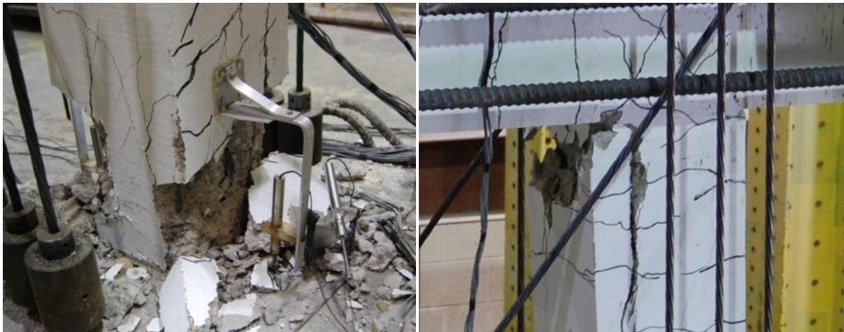
Fig. 4.15 Column damage at 2.5% drift; (a) crushing of column concrete near the base, (b) spalling of column cover near the top joint
