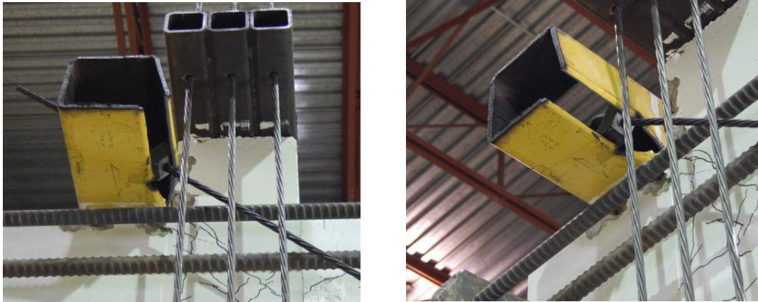
Fig. 4.11 Failure of the HSS section as a result of tendon rupturing
