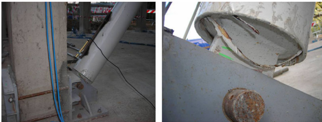
Fig. 2.7 Retrofitted specimen; close-up view (left) and yielding of BRB element (right) - Sarno and Manfredi (2011)
