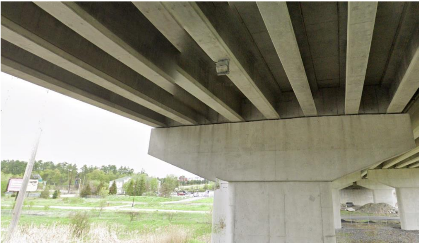
Figure B.4 Closeup Underside View of Overpass Showing Seven Girders Resting on One Pier (Google Maps)
