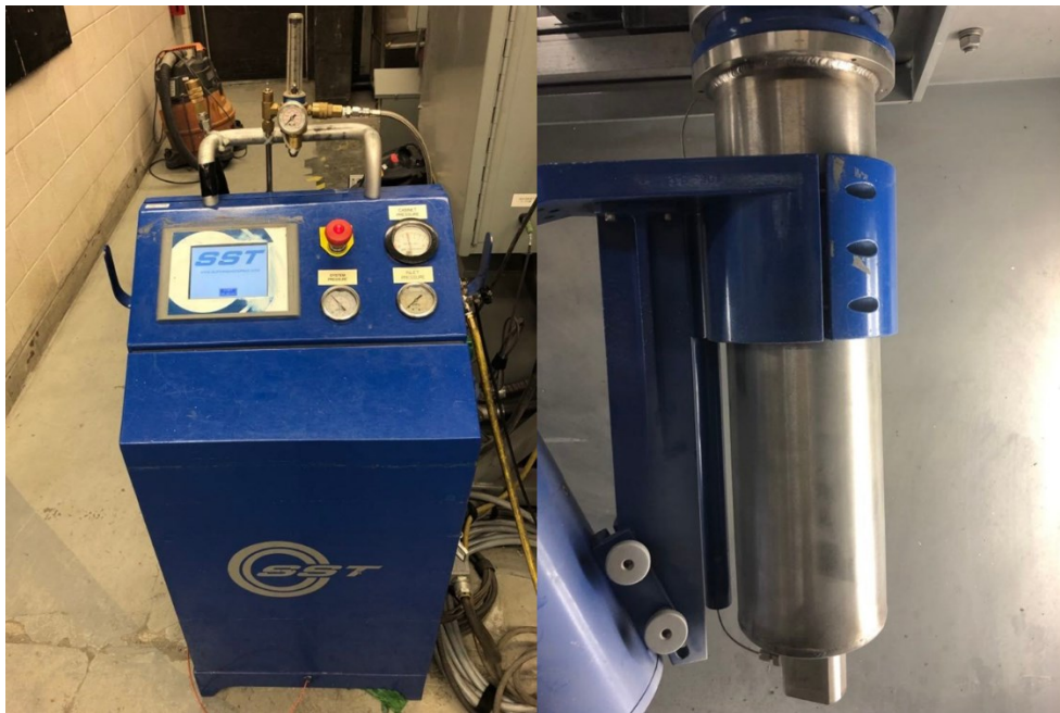
Figure 37. SST control cabinet (left) and gas heater (right)
