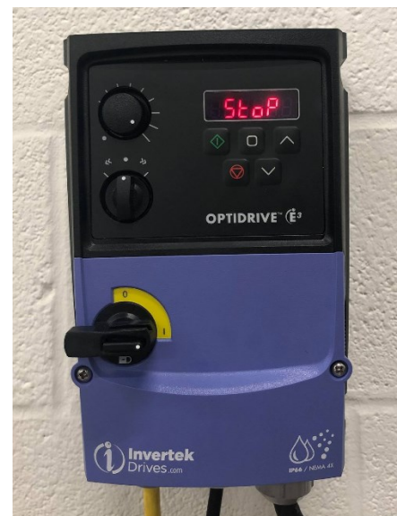
Figure 68. Variable frequency drive unit
