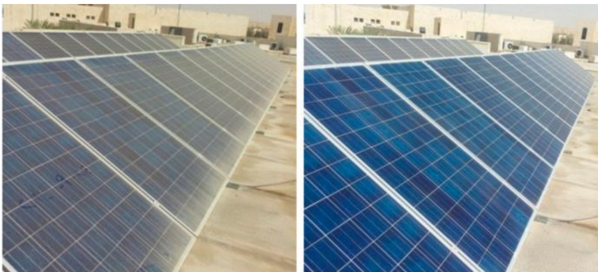
FIGURE 1.4 Dust accumulation on solar panels of an operational solar electric power generation plant. [44]
