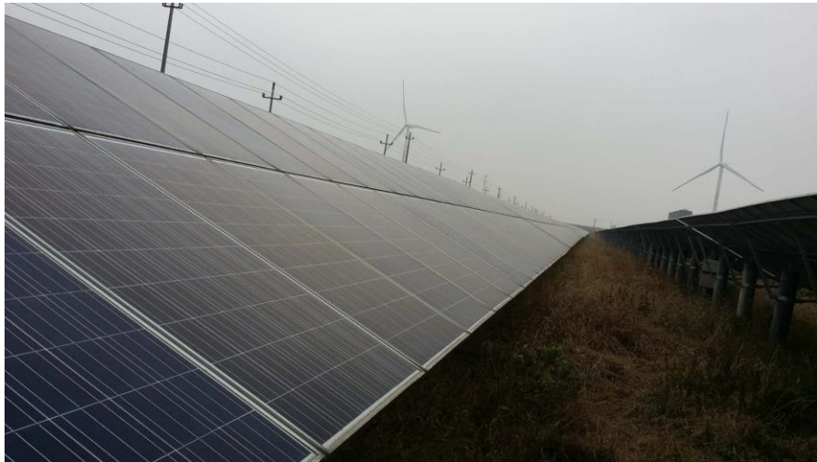
FIGURE 4.3 Typical solar array row at our test site in Jiangshan, Zhejiang, China.
