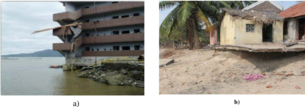
Figure 5-1: Local scour due to tsunami bore around building foundations. a) Japan (courtesy of Dr. Ioan Nistor, 2012); b) 1.4 m deep in India, from the 2004 Indian Ocean tsunami (Yeh and Li 2008)
