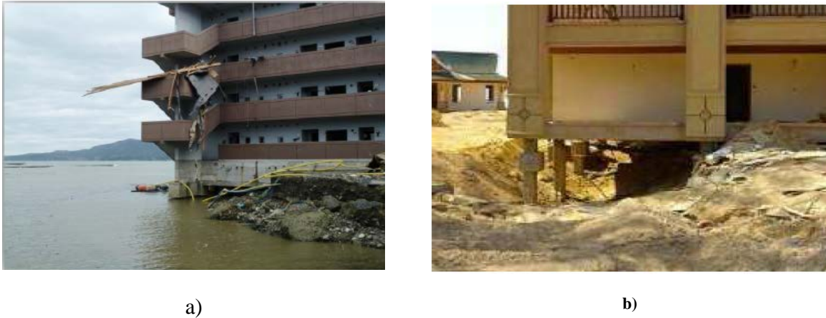
Figure.1: Local scour due to tsunami bore around building foundation a) Japan (courtesy of Dr. Ioan Nistor, 2012); b) Local scour, Koh Khao, Thailand. Case SS-4. Tonkin (2013)
