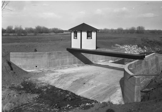
Figure 8: Parshall flume measuring structure, installed[33].
