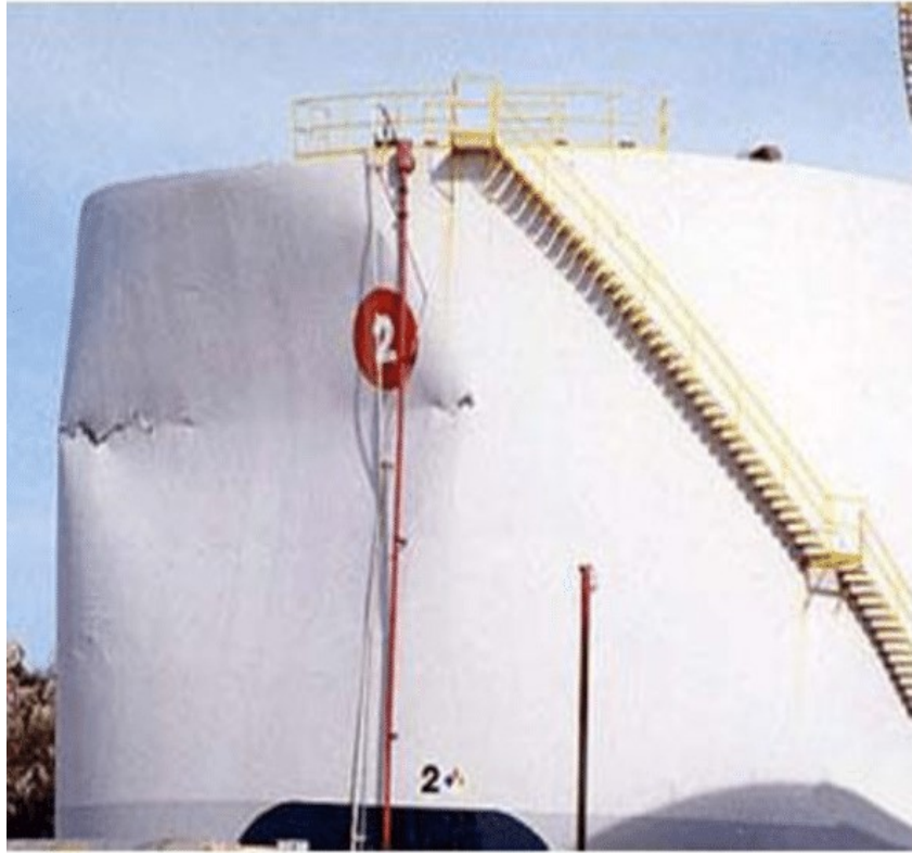
Figure 10: Damage to the tank structure following an earthquake (Source: https://www.researchgate.net/figure/Sloshing-damage-to-upper-shell-of-tank_fig1_336170376 )
