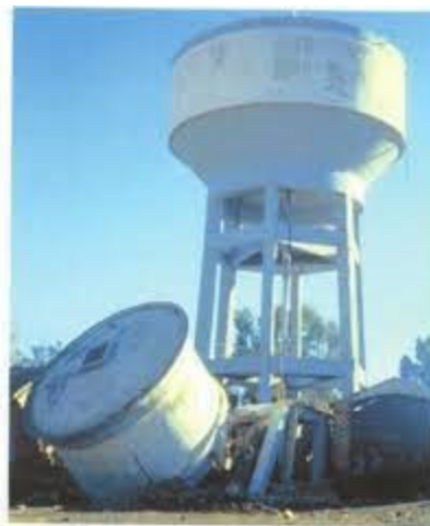
Figure 11: Failure of the reinforced concrete support of a water tank following the 1980 El-Asnam earthquake, Algeria (Source: Soroushnia et al., 2011 [6])
