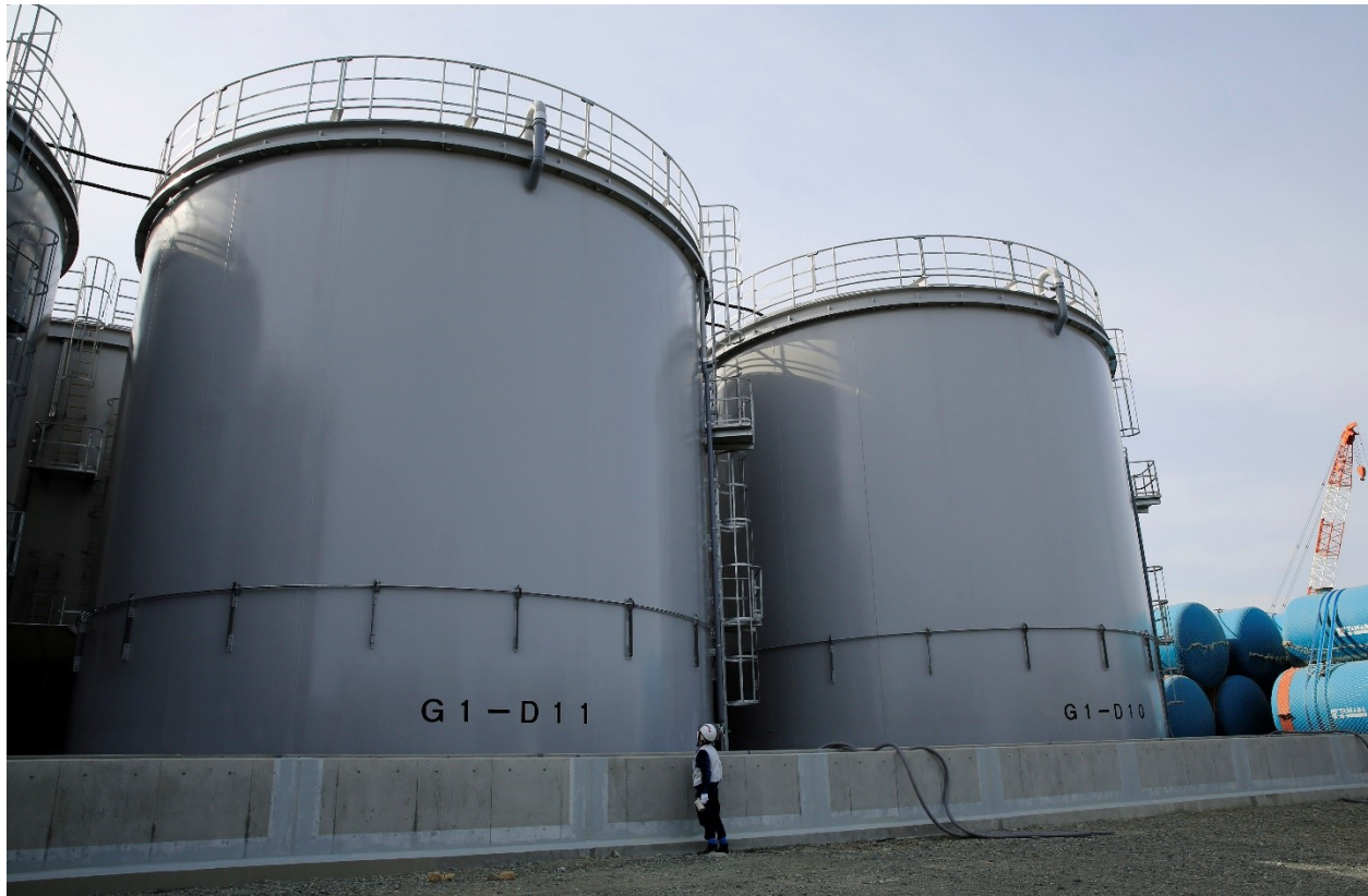
Figure 3: Tanks in a nuclear facility (Source: https://www.reuters.com/markets/commodities/ice-wall-japans-fukushima-nuclear-plant-may-have-partially-melted-nhk-2021-11-26/ )
