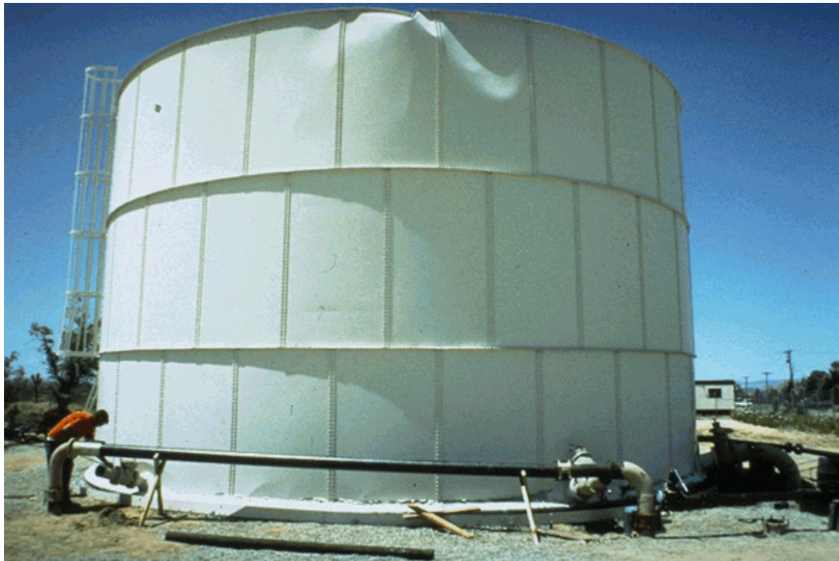
Figure 9: Tank structure damage by the sloshing liquid following the 2010 Landers Earthquake (Source: http://www.johnmartin.com/earthquakes/eqshow/lan_0004.htm )
