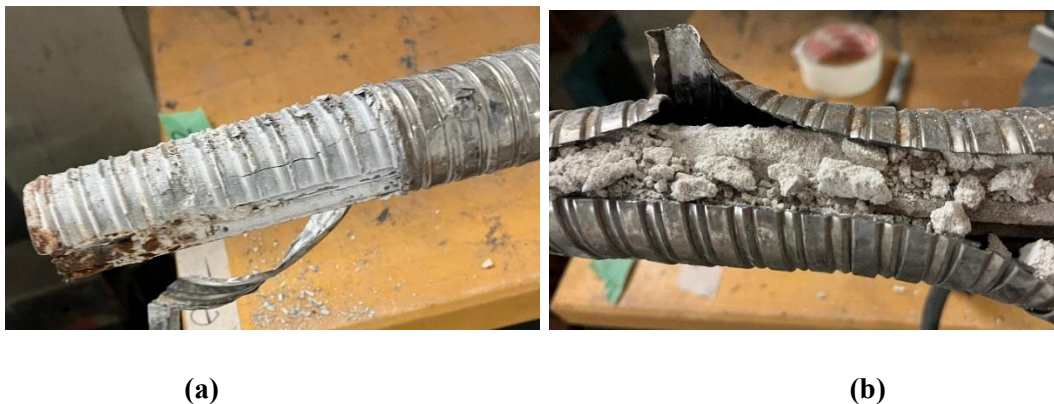
Figure 4-12 Grout conditions in tendon ducts: (a) solid in S5A2-S5B2, and (b) crumbled in remaining tendons
