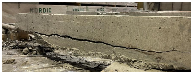
Figure 4-11 Evidence of bond failure in slab S2A3-S2B3
