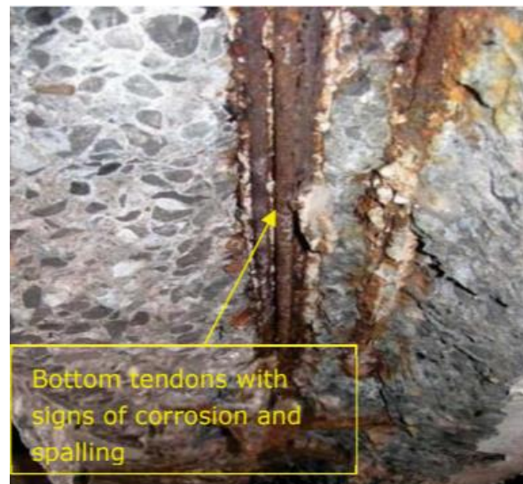
Figure 1. 2- Signs of corrosion in Champlain Bridge (COWI 2017)
