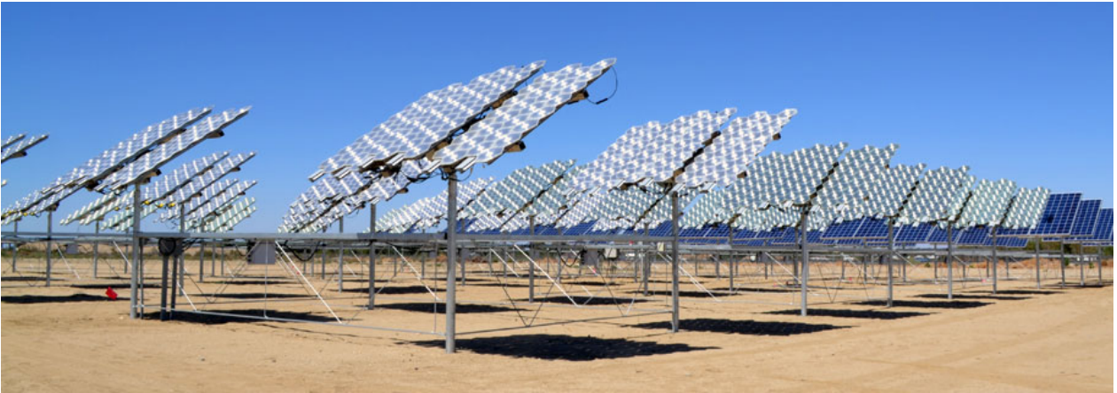
Figure 1.3: Concentrator photovoltaic solar farm with Morgan Solar modules and dual-axis trackers [B - 3].
